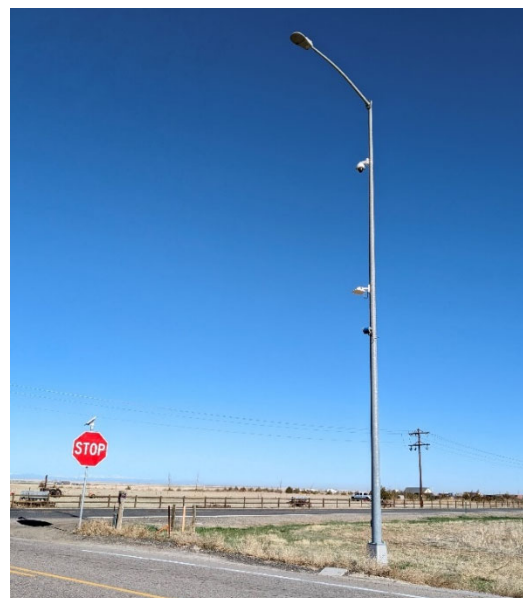
Luminaire with PTZ Camera and Detection
