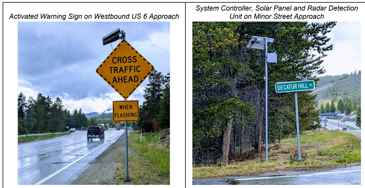
Figure 11: ICWS at US 6 and Saint John Road/Decatur Hill Road, Keystone
