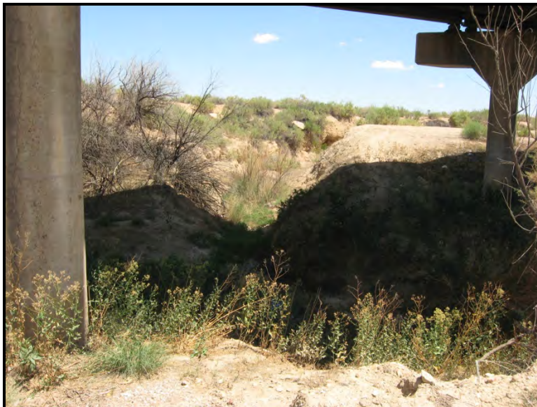
Photo 2 — Looking northeast at an erosion channel north and east of the westbound bridge.
