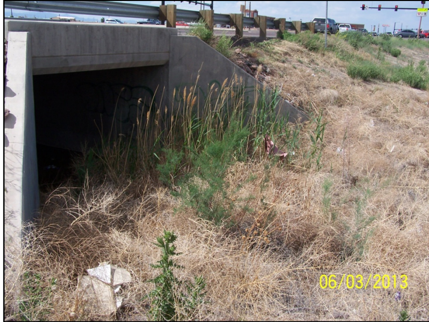
Photo 11 — Looking north next to the box culvert under Purcell Blvd., for the tributary to Williams Creek.
