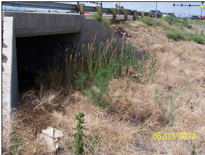
Photo 12 — Looking north next to the box culvert under Purcell Blvd. for the tributary to Williams Creek. This drainage is highly channelized and filled with noxious weeds.
