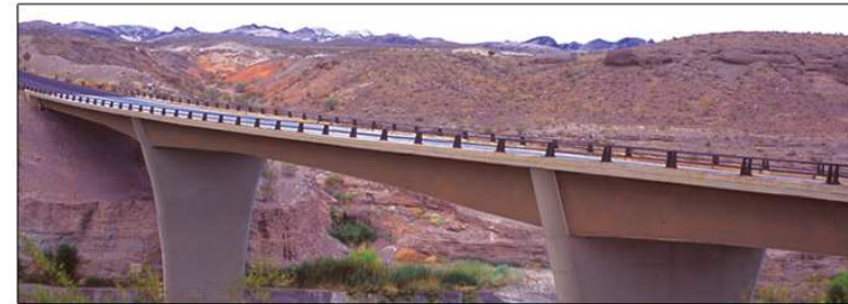
A | Bridges with simple forms, color, and shadow patterns exhibit an aesthetic contrast to the complexity of the natural landscape.
