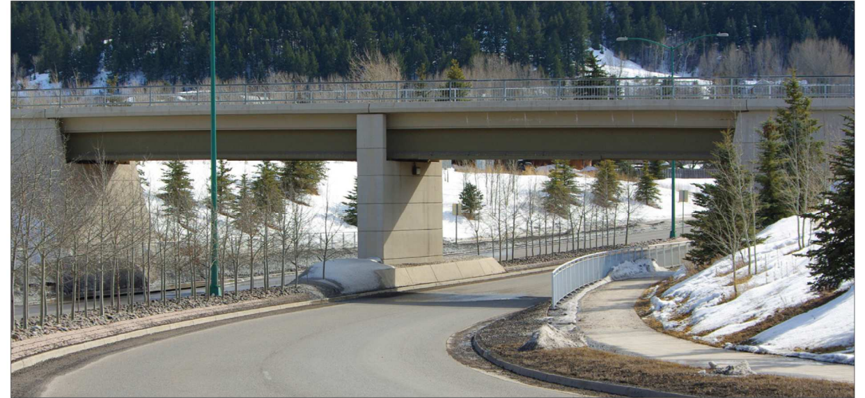
A | Safety and accessibility is improved by open, day-lit connections and a clear separation of vehicular and pedestrian circulation.
