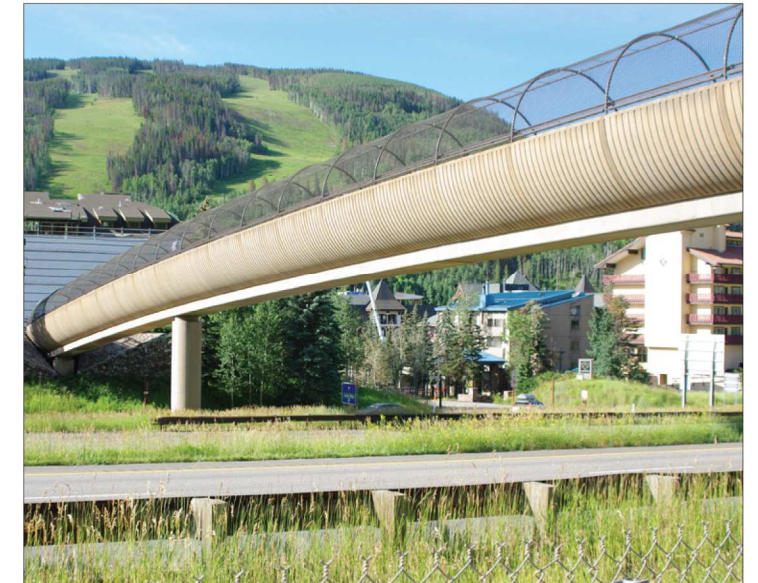
C | Pedestrian bridge crossings reconnect the community when bisected by the roadway.
