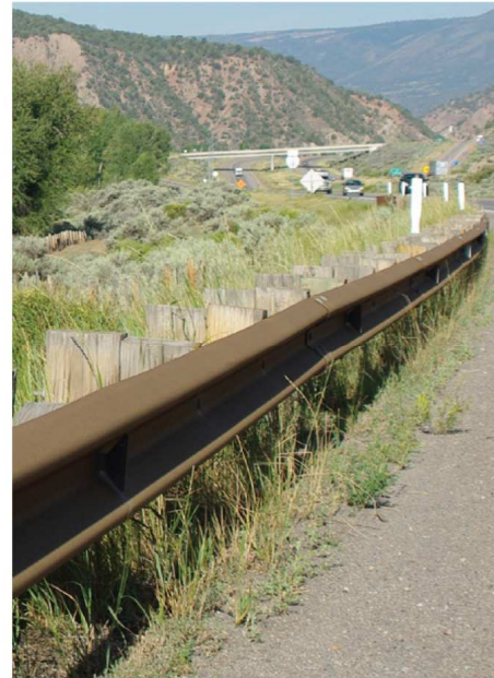
A | Type 3 Guardrail W-beam should be used for guard rails throughout this design segment.
