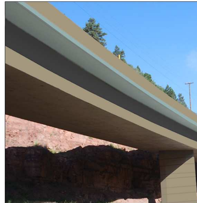
B | Application of segment base color and accent color on bridge structure.
