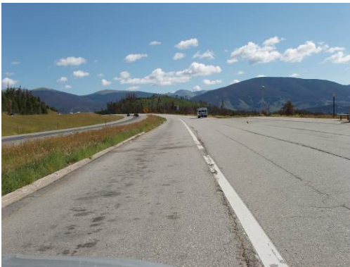
EB MP 203 Chain Station
