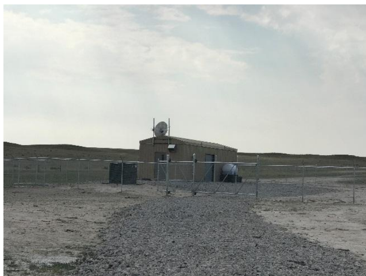
Figure 2. Existing generator and AST in the Study Area
