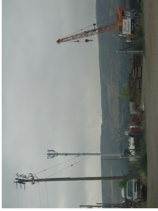
Pascal Construction Co., located north of SH 58 in the northwestern portion of the project area
