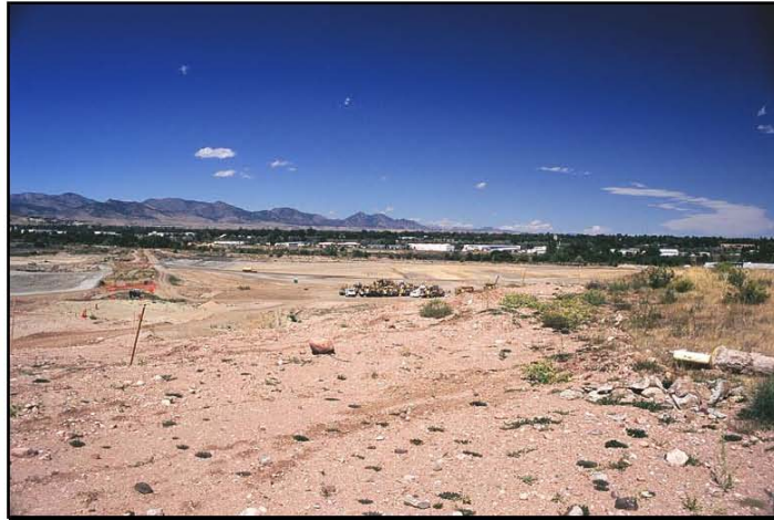
Construction activities occurring on the Coors Everist Parcel on 9/12/2005. This area was surveyed for Spiranthes habitat in 1998 by ERO and again in 2004 by Savage and Savage.
