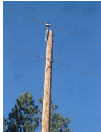
Figure 4-18. Example Electric Pole
