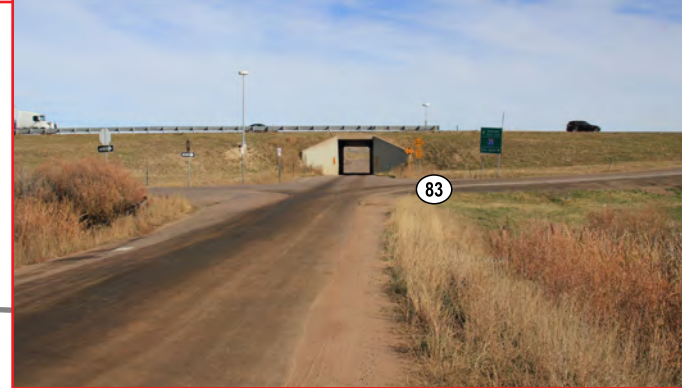
MP 167.5: View from Greenland Road looking east toward the undercrossing of I-25.
