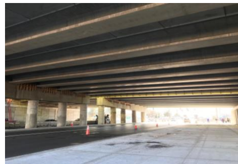
Peoria Street after 12-foot shared-use sidewalks are installed on the east side. The west side has 8-foot walkways.
