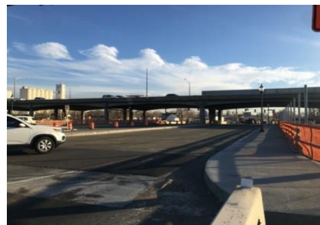
Steele Street after 8-foot sidewalks were installed on the west side. In the future the east side will also have 8-foot sidewalks.
