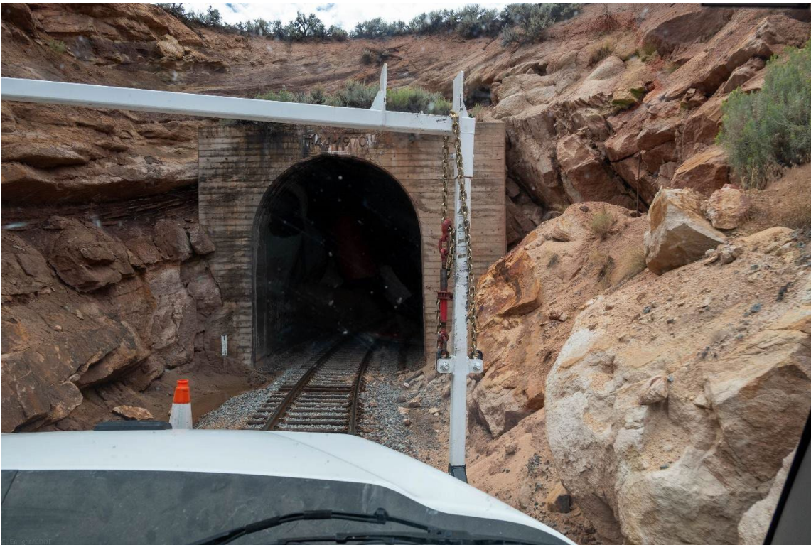
Figure 4: Existing Tunnel 44 with Probable Clearance Issue
