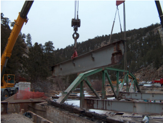
Crews demolish the existing steel truss bridge. The truss will be incorporated into the Town of Estes Park trail system.
