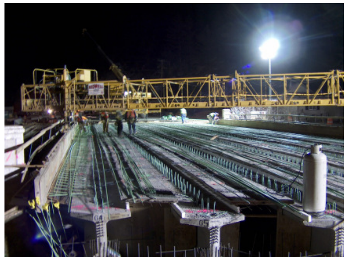
Crews worked 24 hours a day during the closure in order to reopen US 34 to traffic four days early. This particular photo show crews working on the new bridge deck.
