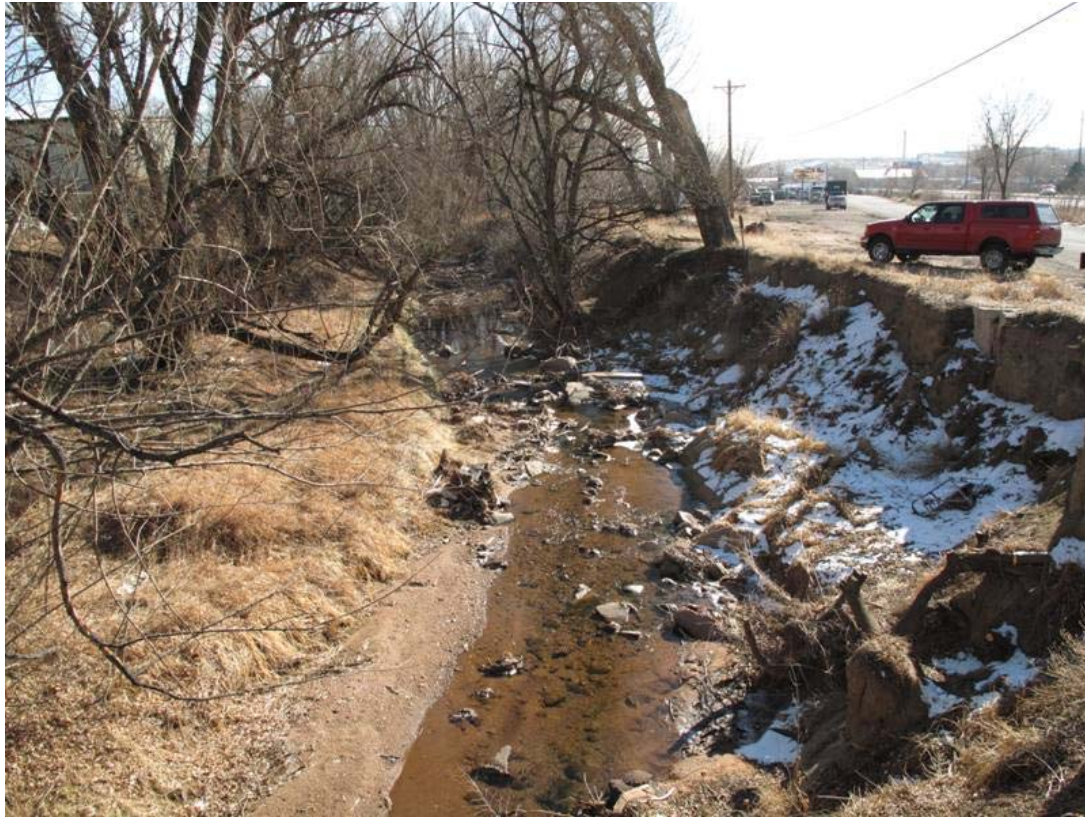
Photo 3: View of erosion along the banks of Fountain Creek near S. 25 th St.
