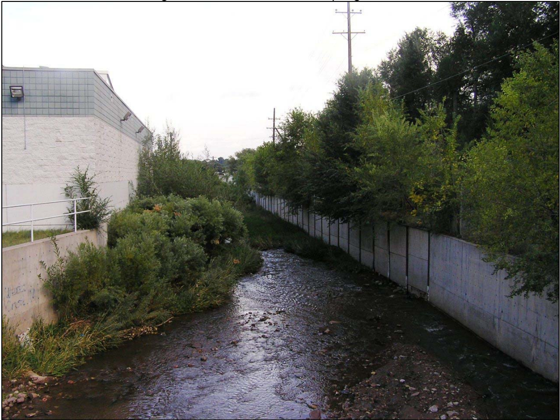
Photo 4. Armored banks present along Fountain Creek, Colorado Springs, Colorado.
