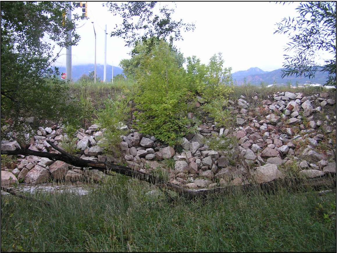
Photo 1. Boulder riprap present along the banks of Fountain Creek, Colorado Springs, Colorado.
