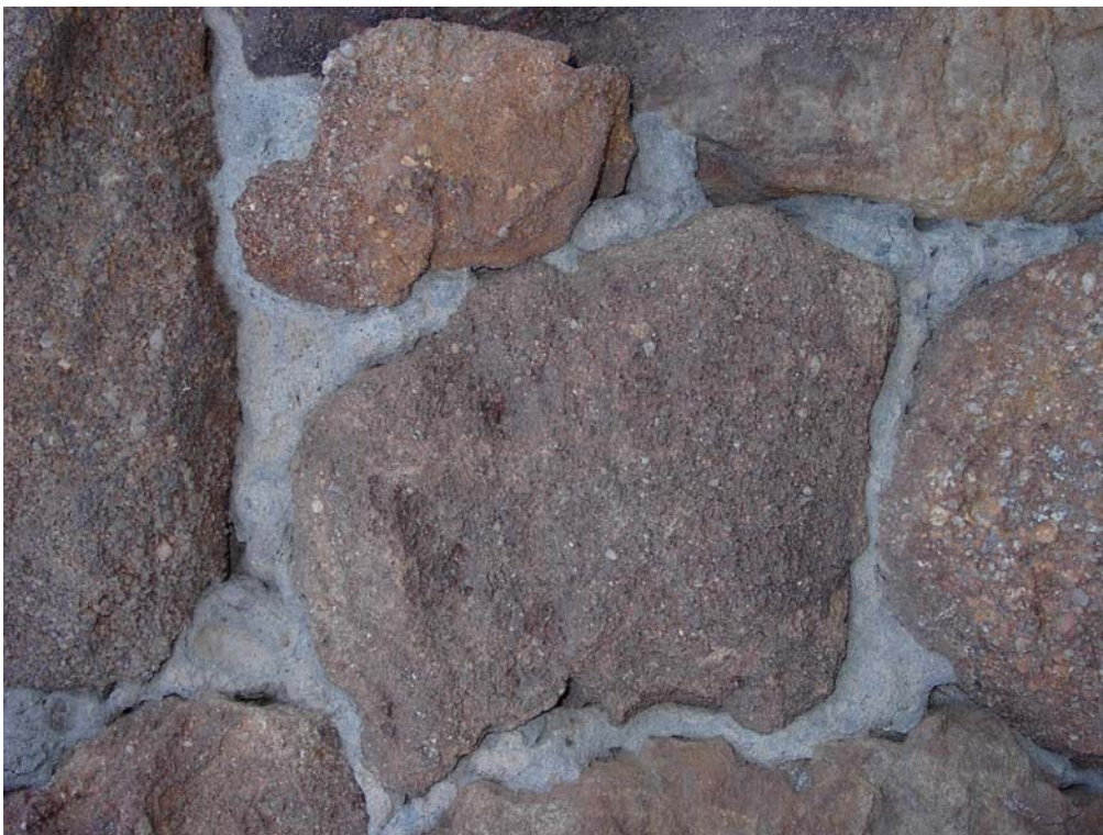
Colorado Springs Monument Valley Arch – Closer view of masonry
