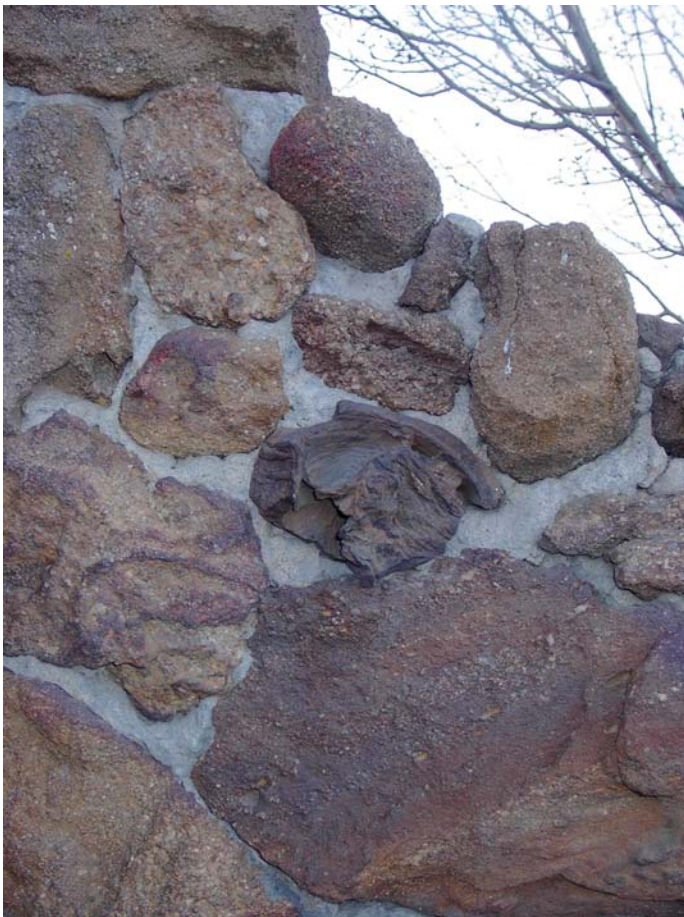
Colorado Springs Monument Valley Arch – Masonry
