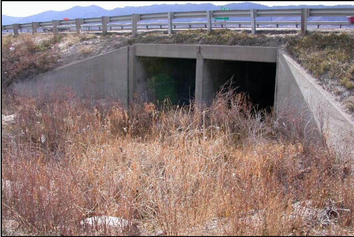
Photo 11. This is the double CBC on the east side of I-25 at Teachout Creek, with a similar structure on the west side. Both structures will be widened. 11/7/02.
