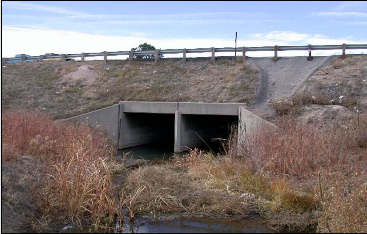
Photo 9. This is the double CBC under I-25 (east side) on Black Forest Tributary. Both ends of the culvert will be extended, causing permanent and temporary impacts. 11/7/02.
