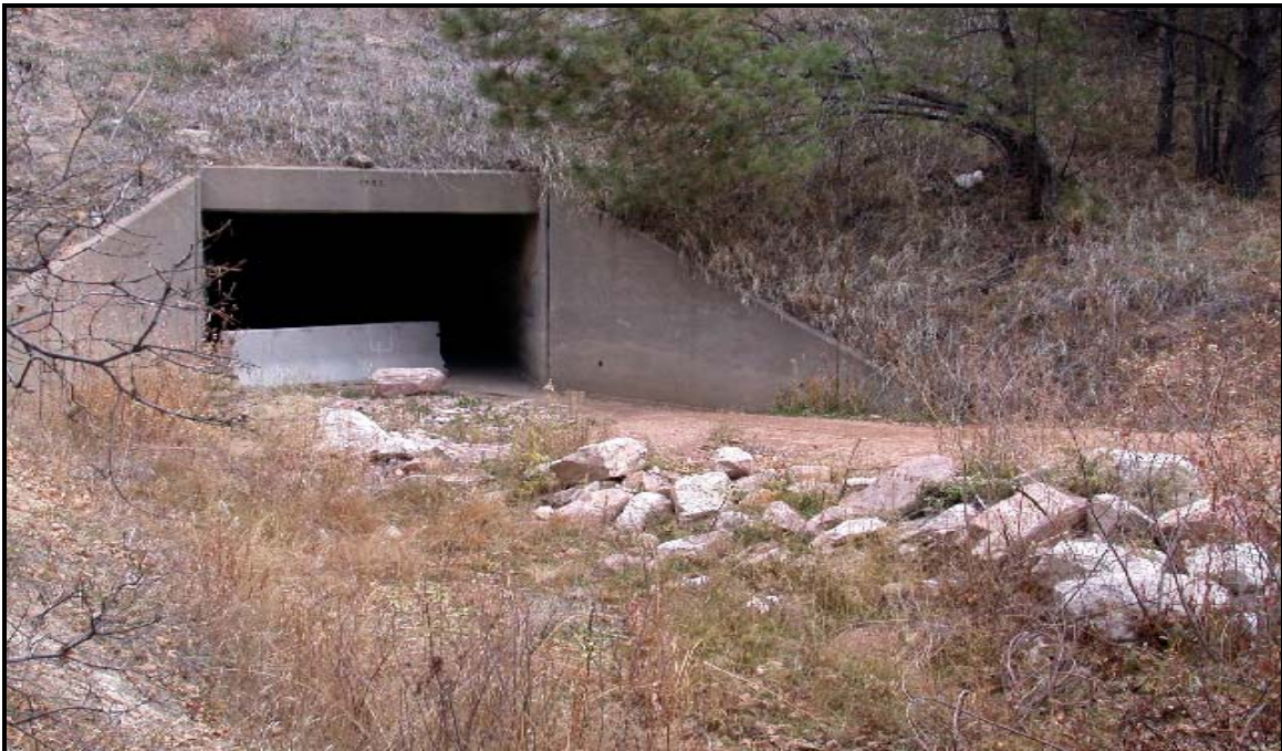
Photo 4. This is the concrete box culvert on Black Squirrel Creek North. Note that the drainage also serves as a trail. The CBC will be replaced and lengthened. 11/7/02.
