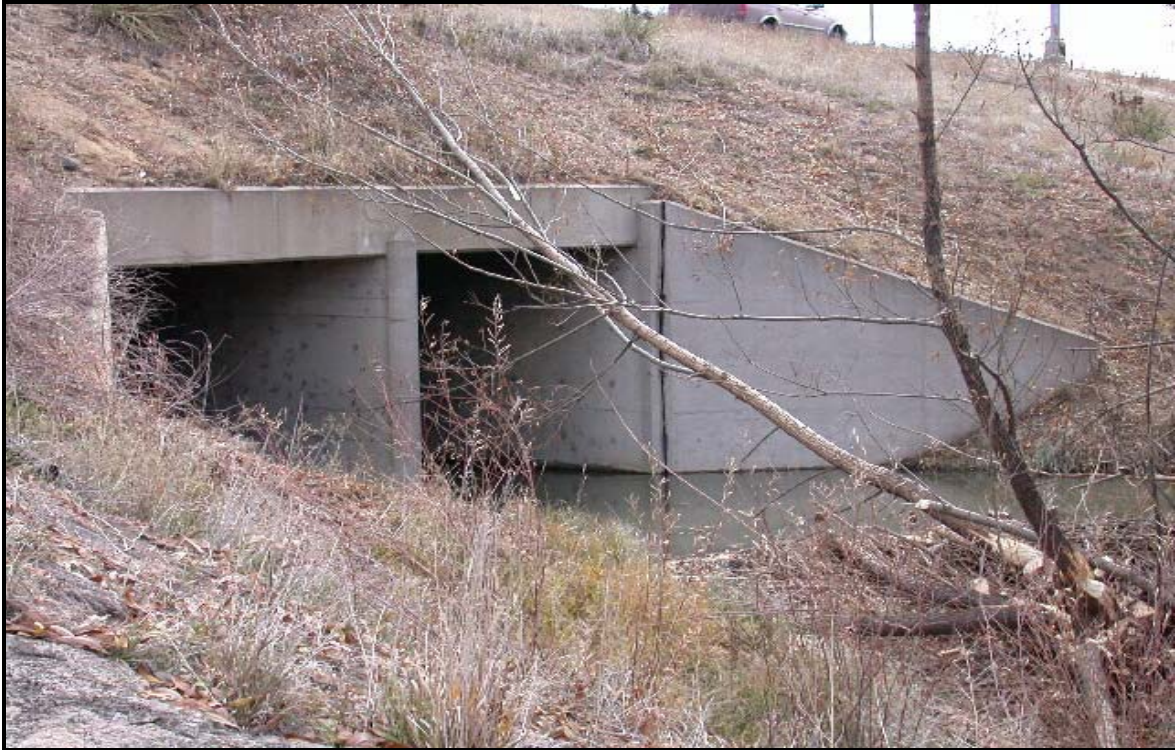
Photo 7. This is the double box culvert under southbound I-25 lanes at Smith Creek (there is a similar structure under northbound lanes). Note recent beaver activity. Both structures will be extended to accommodate roadway widening. 11/7/02.
