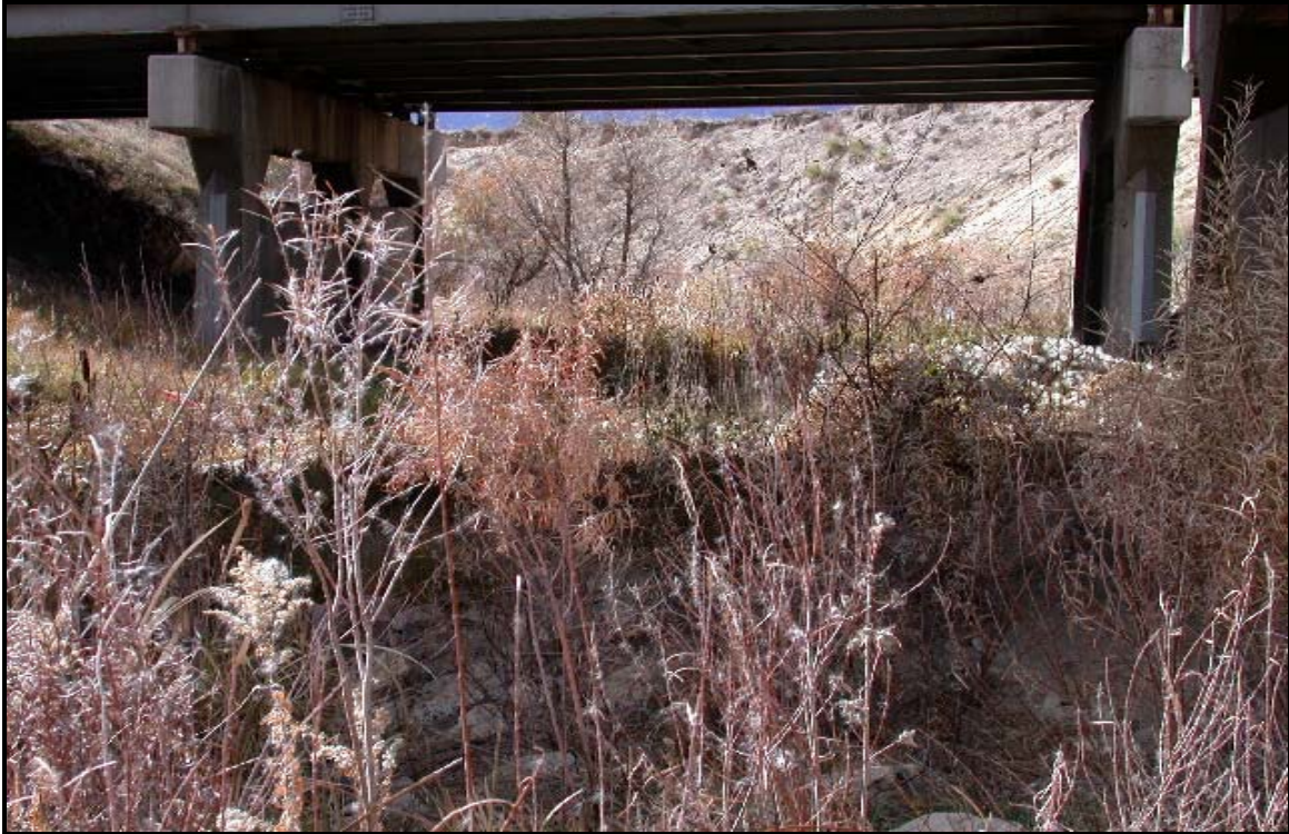
Photo 3. This is the northbound bridge over Black Squirrel Creek South. Both north and southbound bridges will be replaced (new bridges will be widened to the outside), with additional shoulder and embankment work. The open median will remain. 11/7/02.
