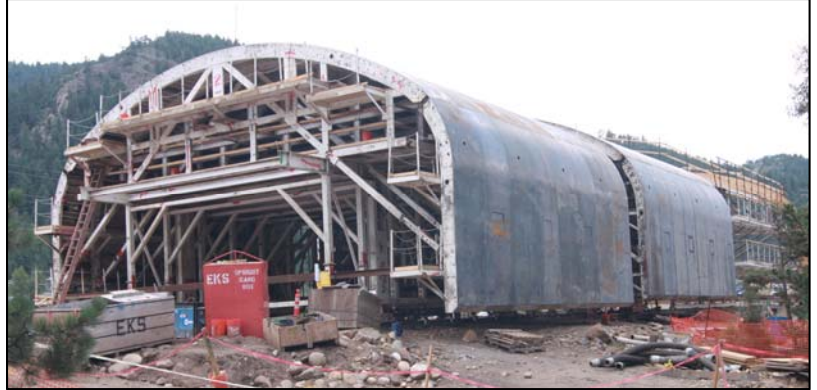
This month, these large tunnel form liner structures will be wheeled into the westbound tunnel bore so work can begin on placing the concrete for the new tunnel lining. Using two of these forms and working from opposite ends of the tunnel, crews plan to do up to four concrete pours a week.
