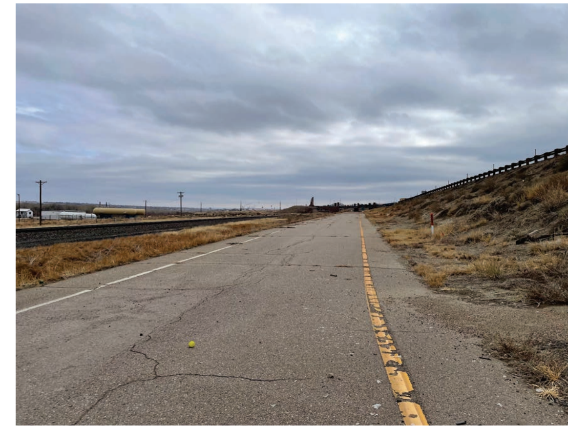
Future location of the I-25 east frontage road near Drew Dix Parkway
