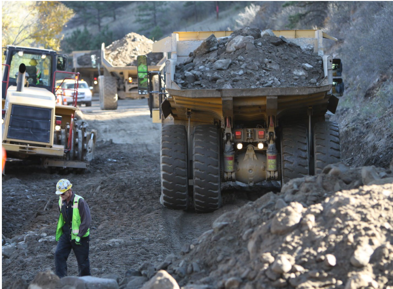
Figure 2 - US 34 Big Thompson Canyon Rebuilt After 2013 Flood
