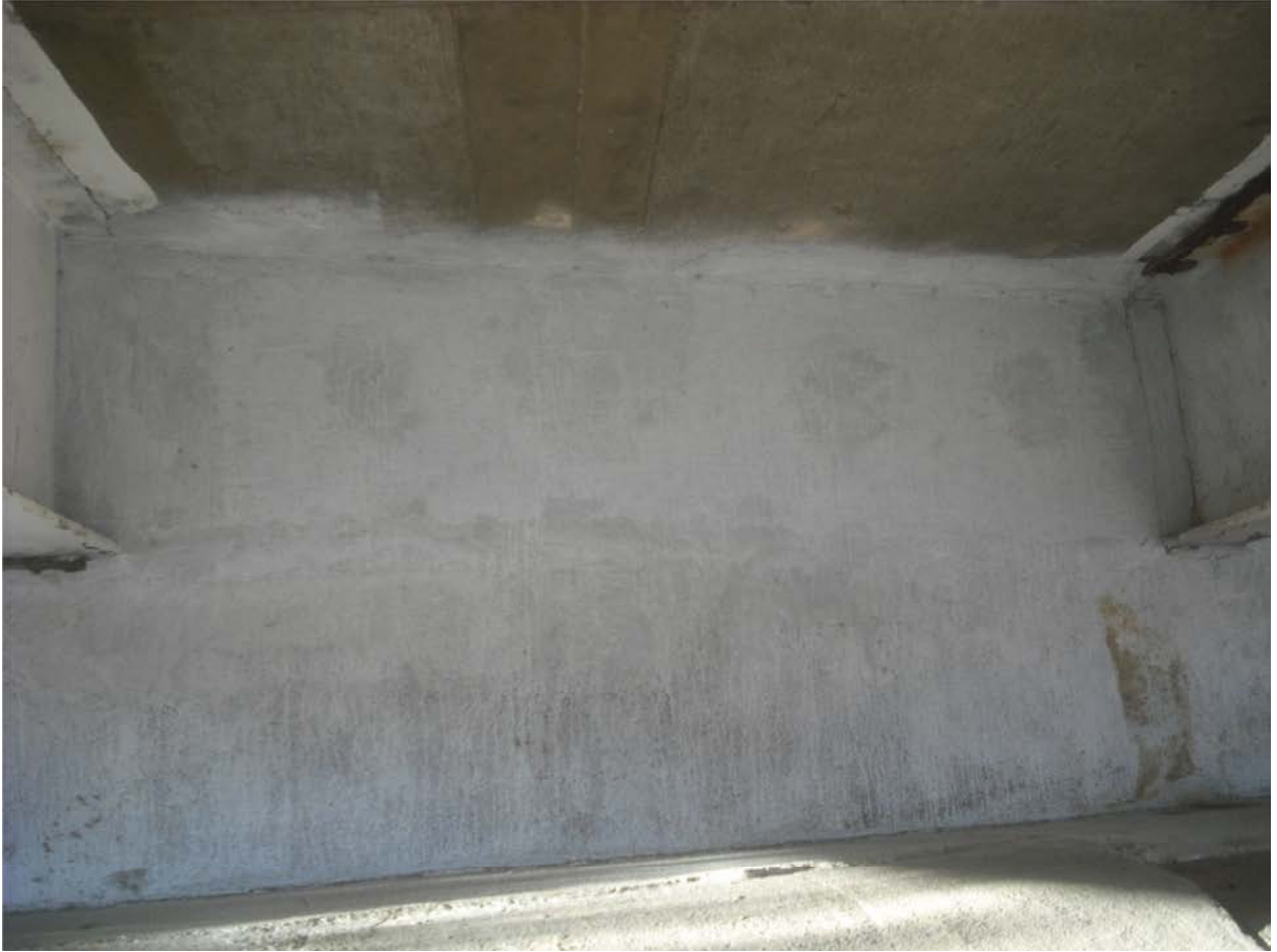
Figure 8: Typical Surface Finish of Normal Concrete
