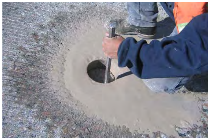
Figure 3-2 Coring concrete samples on Bridge G-22-BJ. It was broken in the traffic lane
