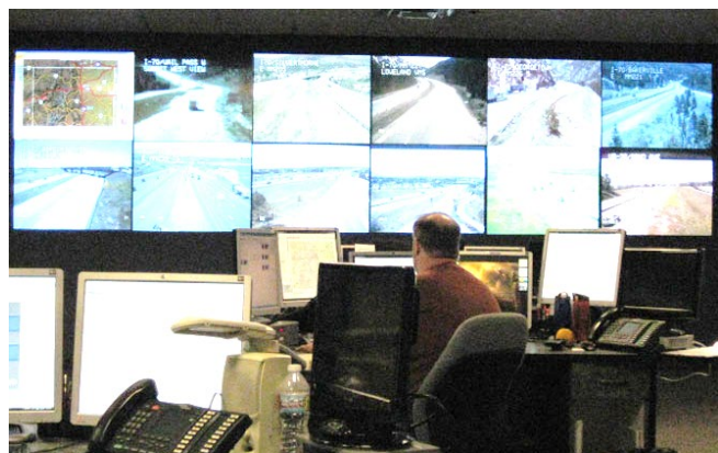
Figure V.9: CDOT Traffic Operations Center
