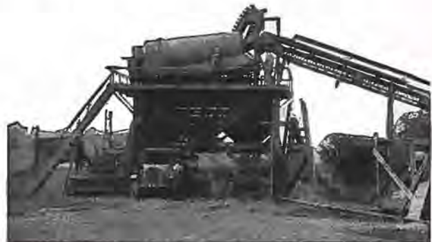
Another view of No. 304-W showing the three compartment bin for sand, pea gravel and coarse aggregate to size called for in specifications.
