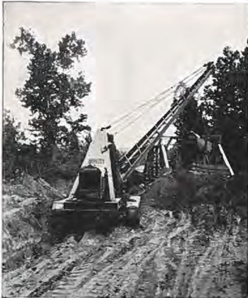
McCormick-Deering Power is operating this shovel, engaged in building approaches to the bridge shown.
