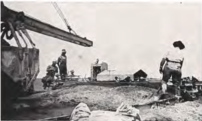
Showing concrete paver and finishing machine in operation on the Selander contract.
