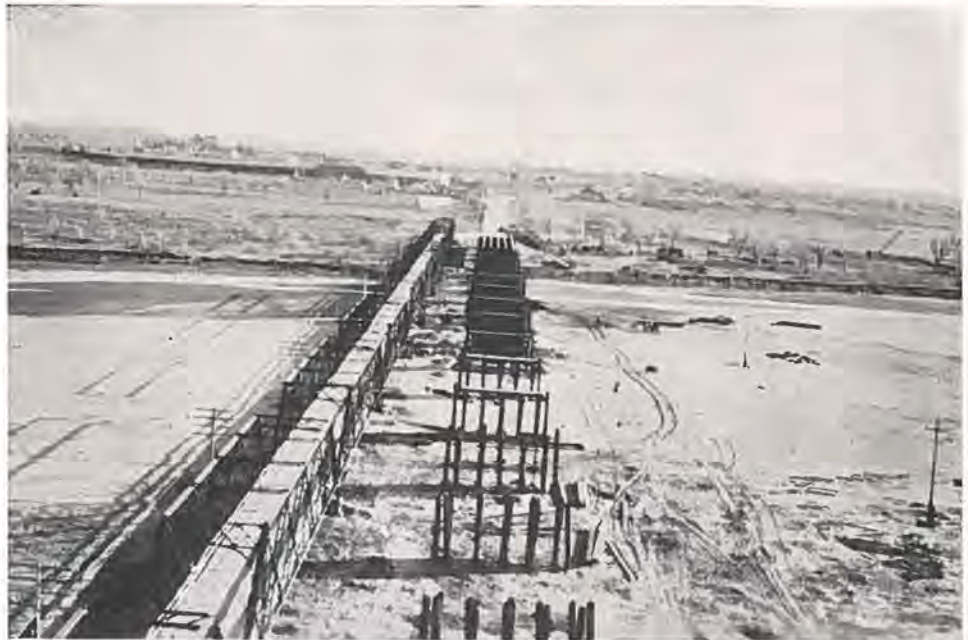
Work in progress on the new bridge across the Arkansas River, near Lamar. Photo shows old bridge moved down stream and now in use as a detour. Photo by L. A. Rose.
