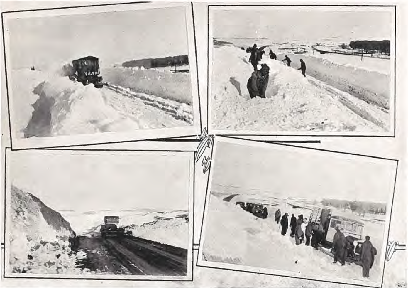
Views showing state highway maintenance crews clearing snow from highway near Limon, following one of the worst blizzards in the history of Colorado. Drifts in places were 20-foot in depth and traffic was blocked for several days. Upper right picture shows crew hand-shoveling snow from roadway. Photos by John P. Donovan.
