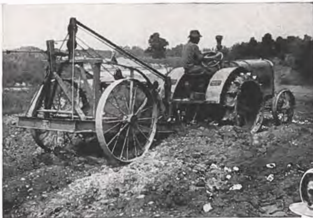
One man can load, transport, and place a lot of dirt in a day with outfits of this type.
