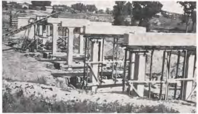
Looking north at substructure for Fountain Creek bridge. When completed this bridge will be 540 feet in length. Photo by Paul Bailey.
