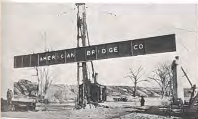
Raising first 80-foot girder in place on new Fountain Creek bridge. Note steam shovel on ice. Photo by Paul Bailey.
