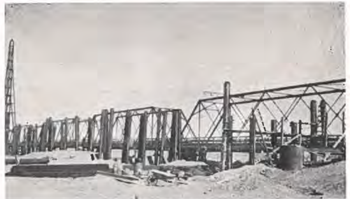
Pile driving for new Lamar bridge, being constructed by Colorado Highway Department with Federal Aid funds. This bridge will be a half mile in length when completed, and replaces an old steel bridge constructed several years ago. Photo by Paul Bailey.
