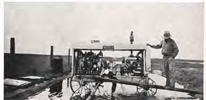
One of the powerful high-speed pumps used for supplying water to mixer and for curing.
