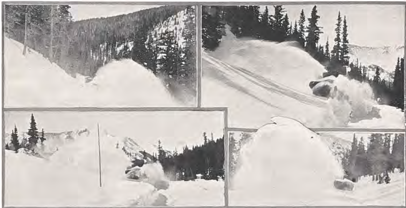
Clearing snow from Berthoud Pass with a giant rotary plow. Twelve miles of snow and ice from 10 to 17 feet in depth is cleared annually from this important link of the Victory Highway, or otherwise known as U. S. Highway Forty, north. Pictures were taken on both sides of the "divide." Picture in left lower corner was snapped at the summit, over 10,000 feet in altitude. The state maintenance forces hope to have this pass open for motor travel by June 1. Photos by George Sharpe.
