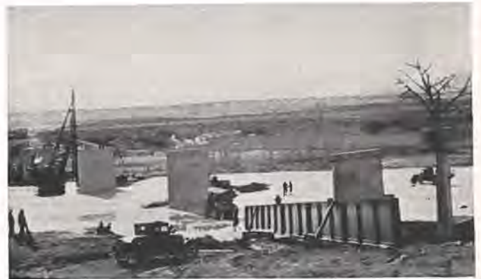
Towing 80-foot steel girder across ice at Fountain Creek, forming link in new highway between Colorado Springs and Pueblo. Photo by Paul Bailey.
