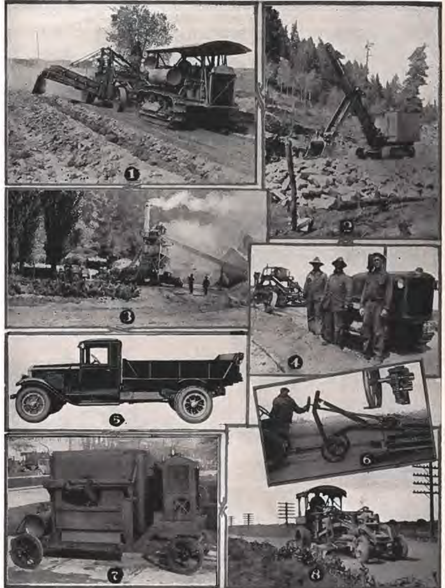
Various types of road building equipment used on Colorado construction and maintenance work. (1) Elevating grader outfit, with Caterpillar tractor, working on new road east of Brush. Photo by Clinton-Held Co. (2) Huge Koehring 1½-yard shovel owned by H. C. Lallier Construction Co. and working on Wolf Creek Pass project. (3) Cedar Rapids pre-mix asphalt plant owned by the H. W. Moore Equipment Co. mixing materials for 2½ miles of oil surfacing south of Glenwood Springs. (4) Monarch tractor crew employed by State Highway Department. (5) New model International contractor's truck. (6) Showing new type No. 61 Adams maintainer. Photo by Elton Fair Company. (7) Chausse portable sand drier and oil mixing plant. (8) Galion one-man maintainer, operating on Pueblo-Colorado Springs highway.
