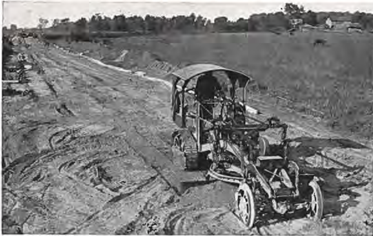
McCormick-Deering - powered grader preparing the road bed ahead of the paver. McCormick-Deering is the power heart of this and countless other types of equipment.
