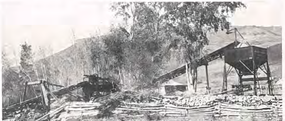
Pioneer gravel crushing plant used by Cole Bros. on Federal Aid project located west of Sapinero. Picture submitted by Elton T. Fair Company.
