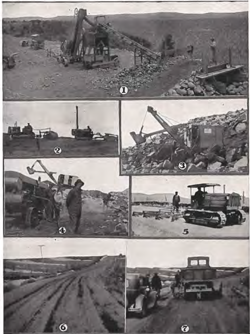
Equipment being used on Colorado road projects: 1. A Pioneer gravel crushing plant owned by Montrose County working near Naturita. Photo by Elton T. Fair Co. 2. A pair of Caterpillar tractors pulling Ateco hydraulic scrapers to crush gravel for project east of Denver. Photo by Clinton-Held Co. 3. Here we have a General excavator working in 13,000 ft. altitude on Mount Evans. Photo by George Meffley, of H. W. Moore Equipment Co. 4. A giant Schramm compressor running two jack-hammers on Mount Evans road project, 13,882 ft. altitude. Photo by H. W. Moore Equipment Co. 5. A Monarch "30" with drag operating on state highway south of Pueblo. Photo by Wilson Machinery Co. 6. Before and After—with an F. W. D. truck equipped with a Willett scraper in Weld County. Photo by Liberty Trucks & Parts Company.
