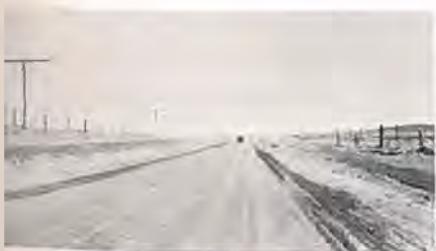
Ingleside Highway between Ft. Collins and Laramie—another excellent example of "Mixed-in-Place" road construction using Midwest (Standard) Asphalt Road Oil.
