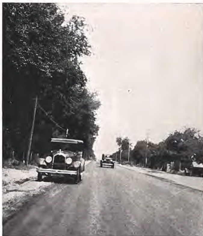
A stretch of the new oil process surfacing recently completed near Canon City.
