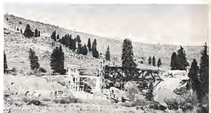
Eliminating a bad "kink" in road between Gilman and Minturn with bridge and overhead railroad crossing.
