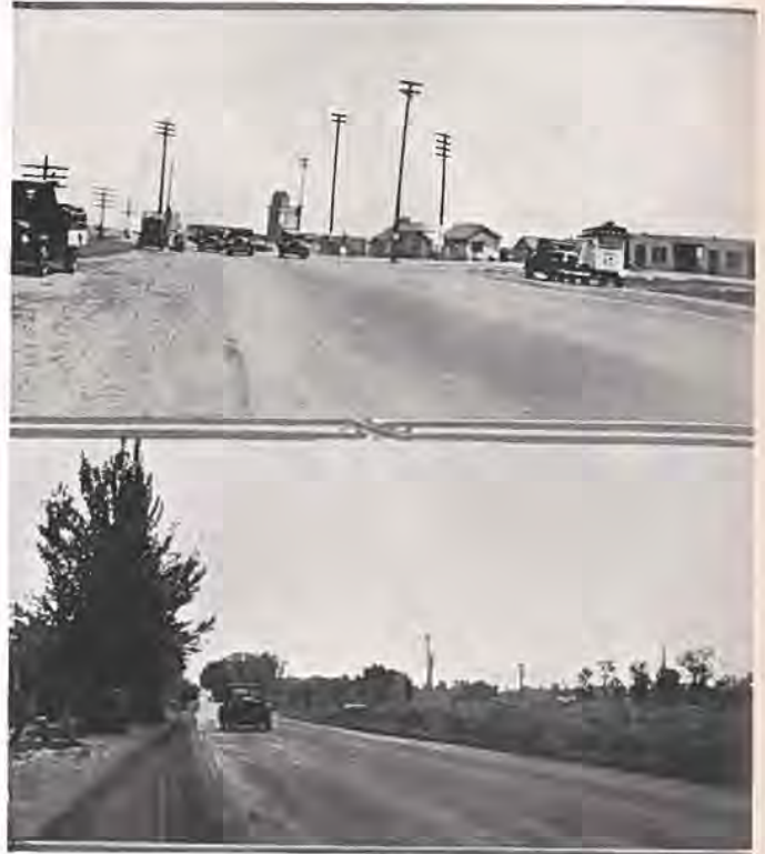
Upper picture shows "mat" method on street connecting with the Brighton paved state highway. Lower photo shows "mixed-in-place" oil processing on Santa Fe Drive.
