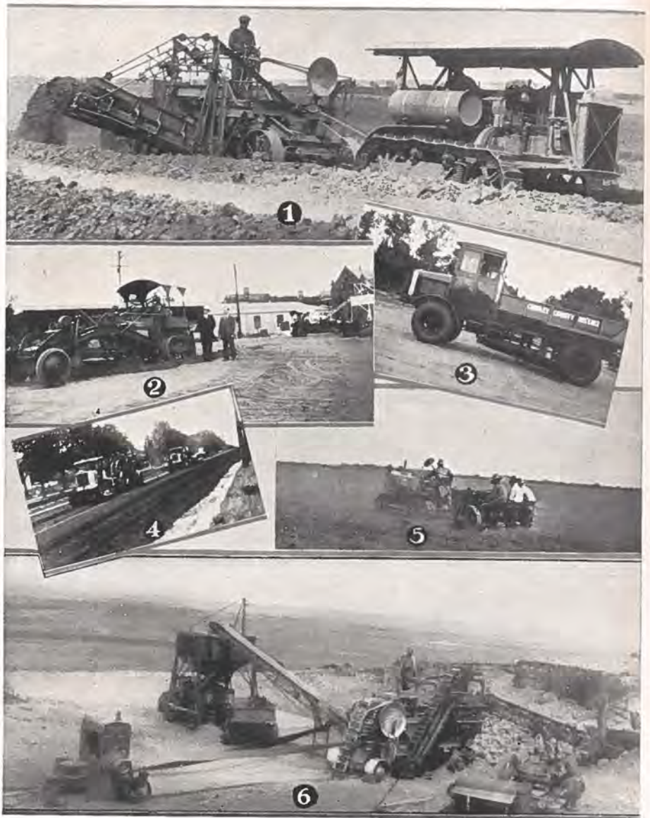
(1) An elevating grader outfit at work in Bent County. Photo by Clinton & Held. (2) One of the new sure-trac Galion one-man maintainers purchased by Baca County. Photo by H. W. Moore Equipment Co. (3) Here we have a photo of a FWD utility truck equipped with Willett Spring scraper, purchased by Crowley County. Photo by T. W. Monnell of Liberty Trucks & Parts Co. (4) Two Bates tractors in use on oil process work near Littleton. Photo by George Meffley. (5) A Cletrac "thirty" used by L. C. Schutte, the U. S. potato champion, near Monte Vista. (6) Pioneer portable rock crushing plant of the Mountain States Construction Co. near Greenhorn.
