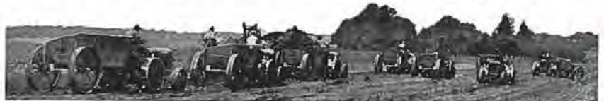
A fleet of McCormick-Deering Industrial Tractors and dump trailers moving dirt quickly and at low cost on a new road in Missouri.
