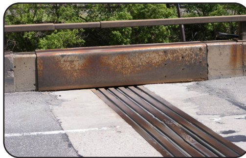
Image 16. Bridge Joint and Rail (F-08-AR)
