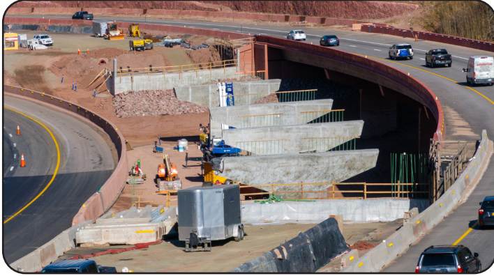
Image 34. New I-70 WBND Structure and Substructure Units for the New I-70 EBND Structure
