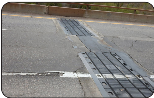
Image 15. Patch to Bridge Joint (F-08-AD)
