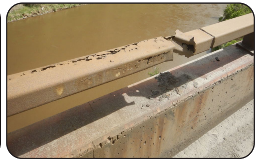
Image 17. Deteriorating Rail (F-08-BJ)
