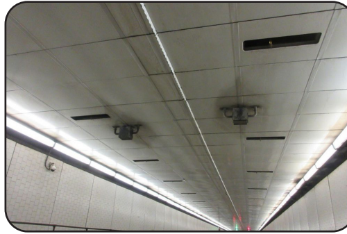
Image 11. Lighting in the Eisenhower Memorial Tunnel
