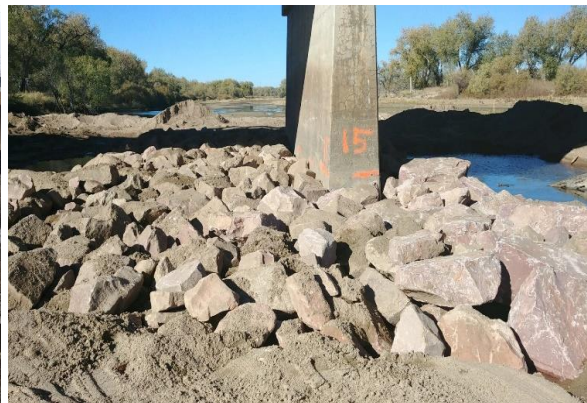
Photo 17.2 Rock riprap installed as pier-scour countermeasures at US 6 in the South Platte River near Merino, Colorado.
