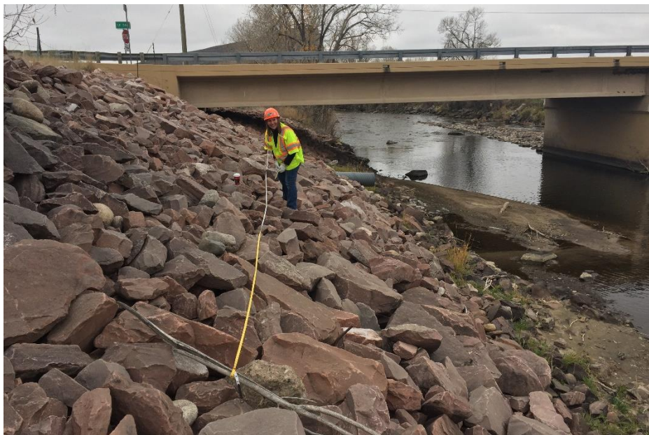
Photo 17.5. Collecting Wolman Counts of post-construction rock riprap at the Cache la Poudre River adjacent to US 287, Larimer County, Colorado, at MP 355.
