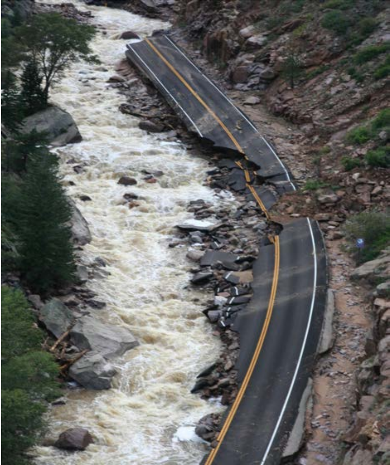
Figure 36 - MP 26.9, Roadway undermined and washed out embankment.
