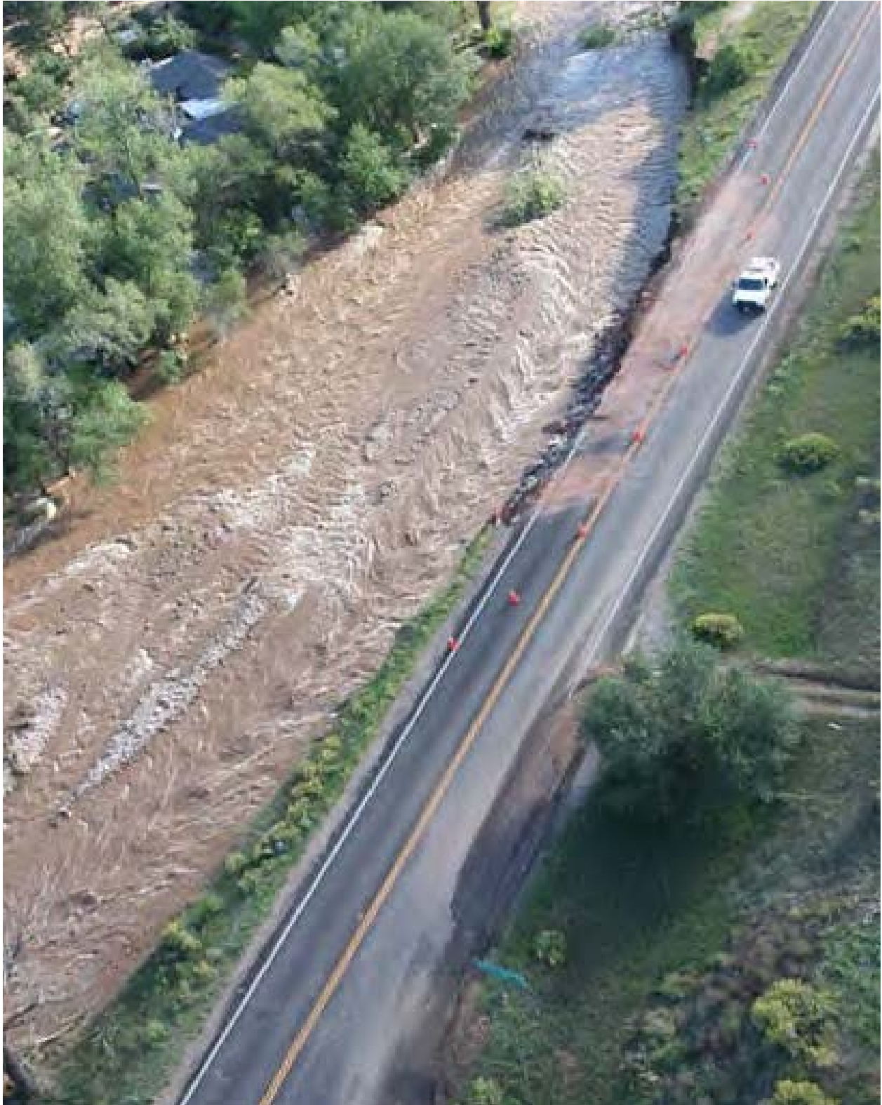
Figure 66 - MP 32.7, Riverside embankment washout and undermined paved shoulder.
