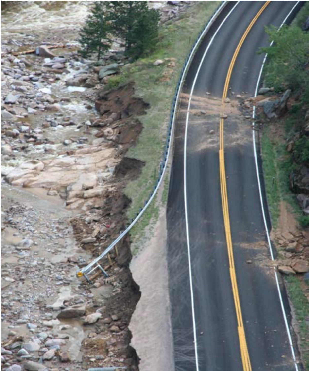
Figure 40 - MP 28.3, Scour damage to gravel pullout, EB embankment and guardrail; and material slides.
