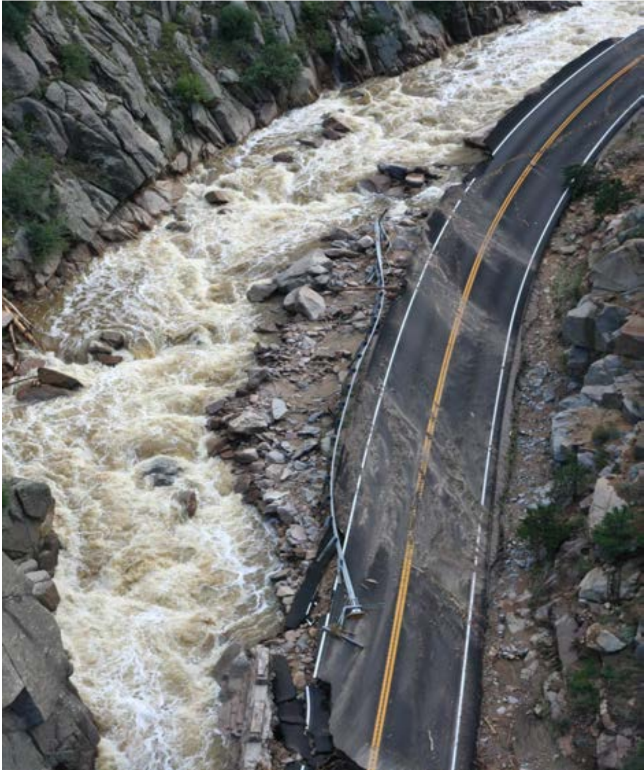
Figure 38 - MP 27.61, Riverside embankment and eastbound lane damage due to lateral scour and overtopping of the roadway.
