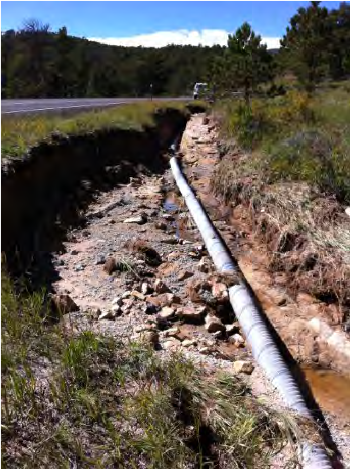
Figure 9 - MP 19.15, Eastbound ditch damage.
