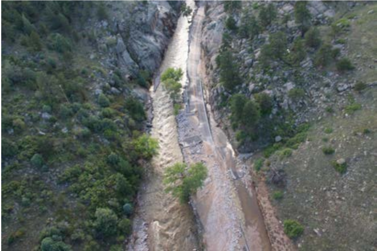
Figure 42 - MP 30.08, Wash out of the roadway embankment and pavement due to lateral scour and overtopping of the roadway. Sediment and debris deposition throughout.
