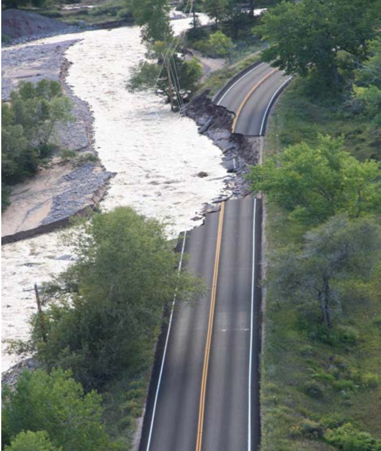
Figure 44 - MP 30.49, Complete roadway loss
