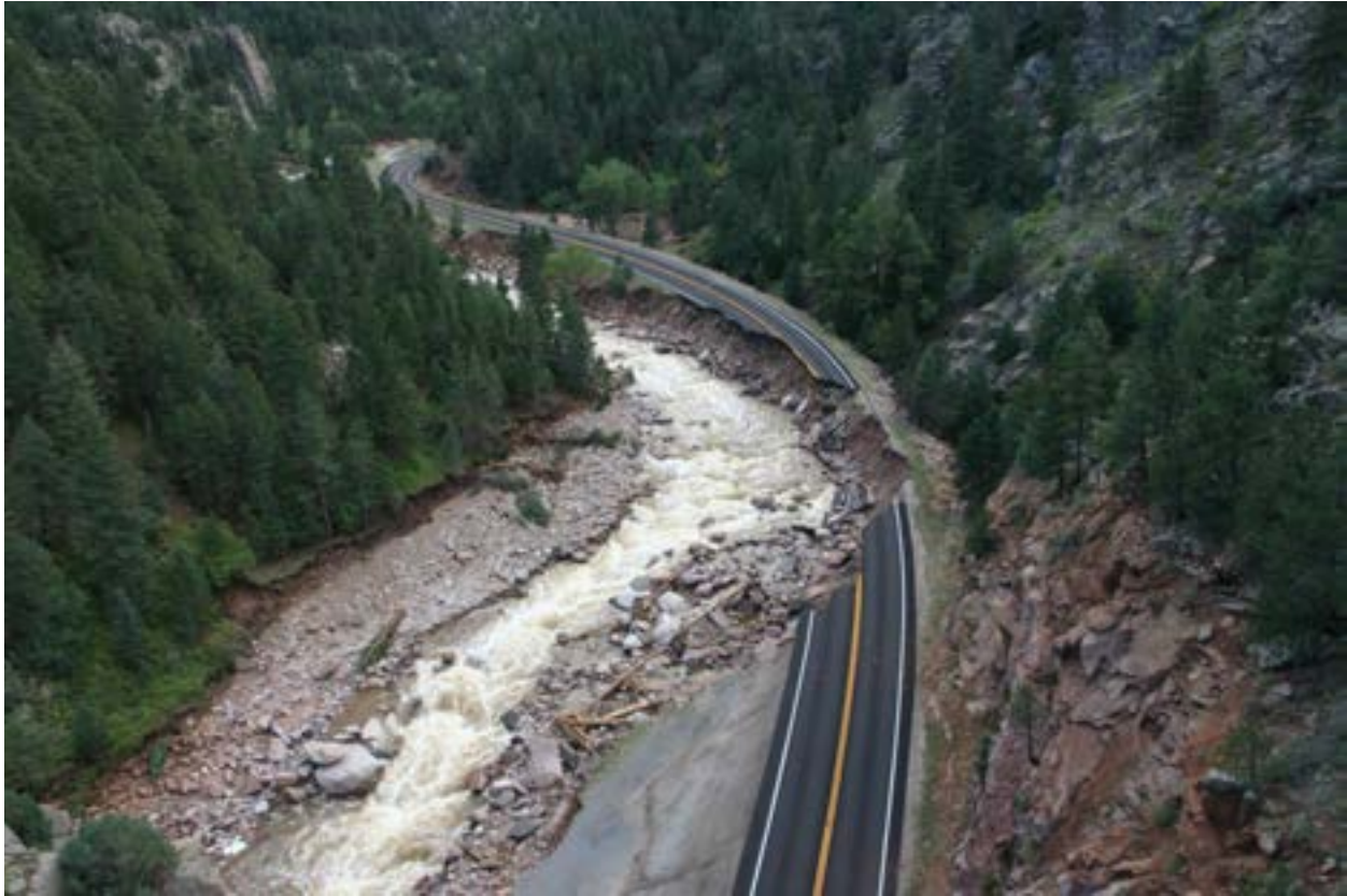
Figure 37 - MP 27.28, Complete roadway loss due to embankment scour damage at the river bend.
