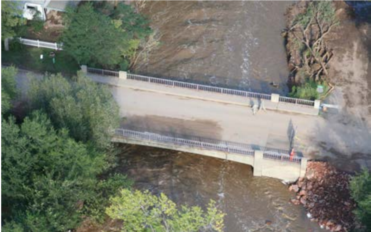
Figure 77 - MP 32.98, Structure D-15-A with abutment scour and undermined pavement behind abutment.
