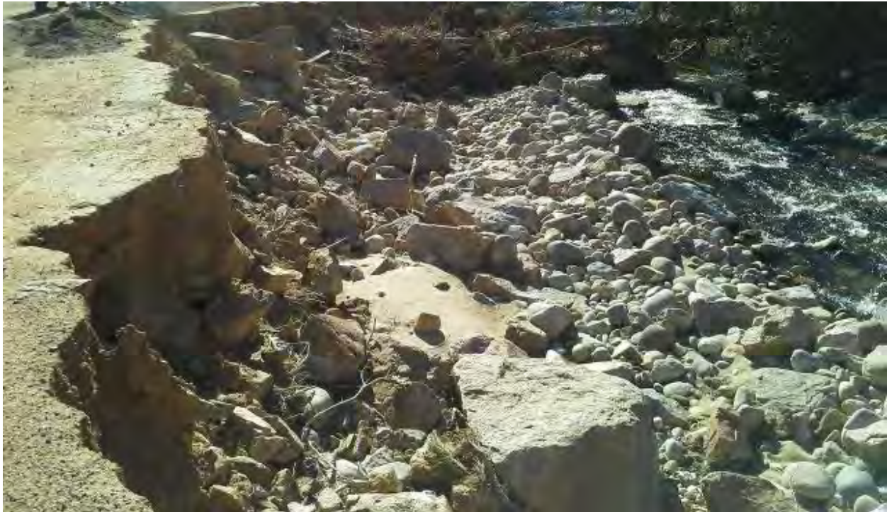
Figure 17 - MP 22.13, Eastbound roadway embankment scour damage.
