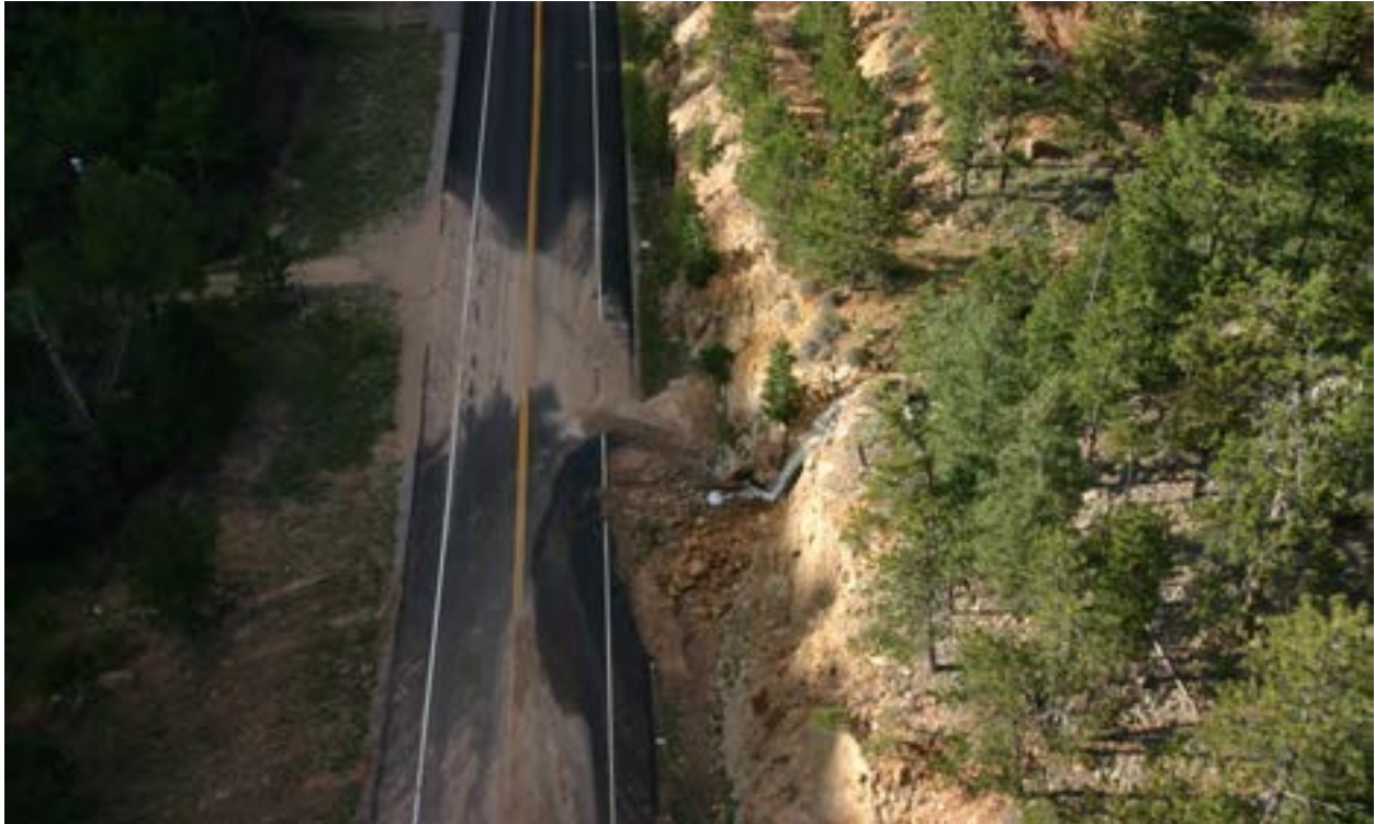
Figure 13 - MP 21.68, Material slide onto road.
