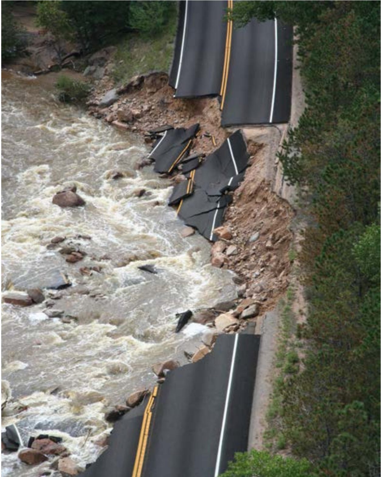
Figure 30 - MP 25.5, Embankment and roadway washout.
