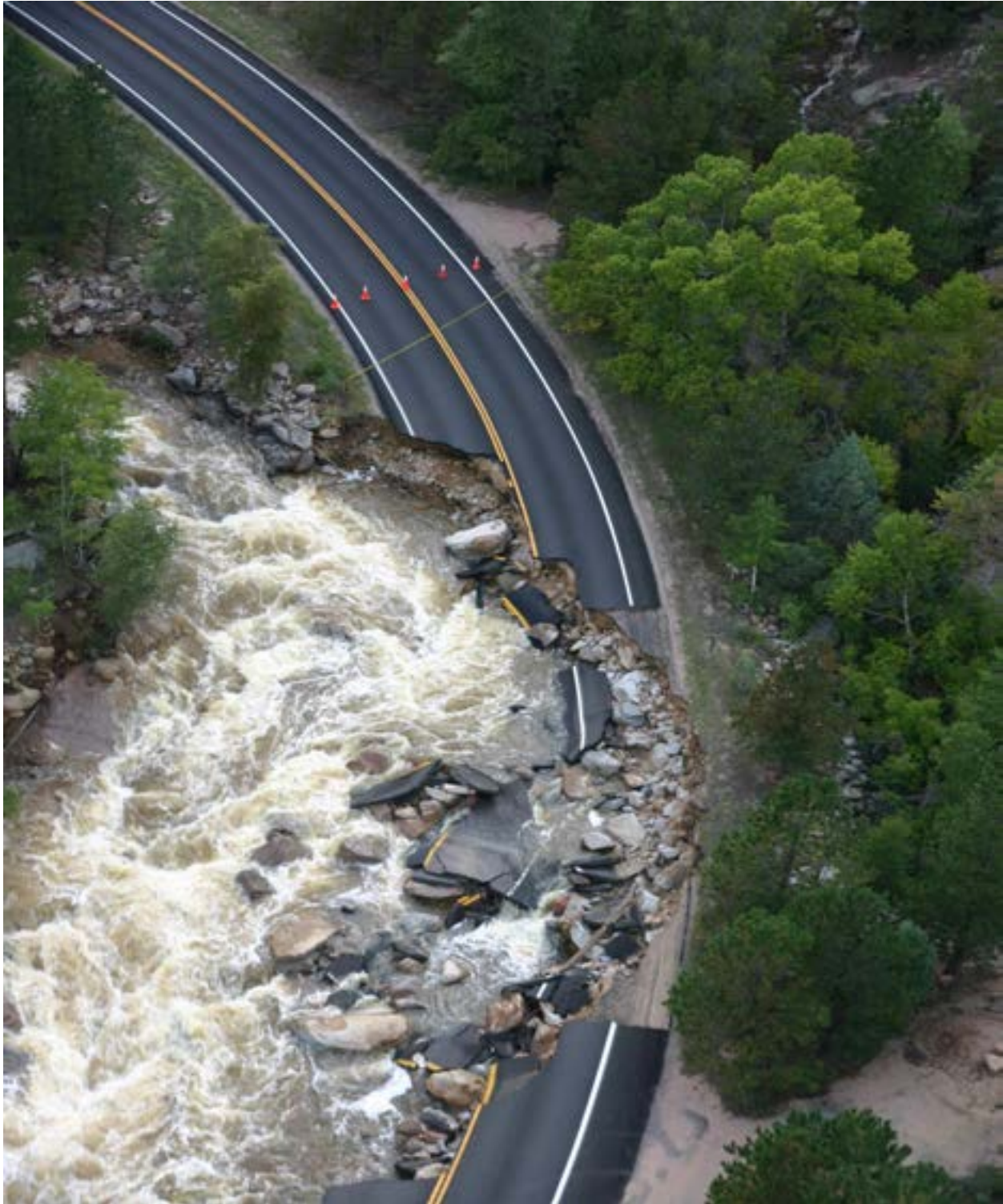
Figure 25 - MP 23.8, Complete 2 lane roadway wash out.
