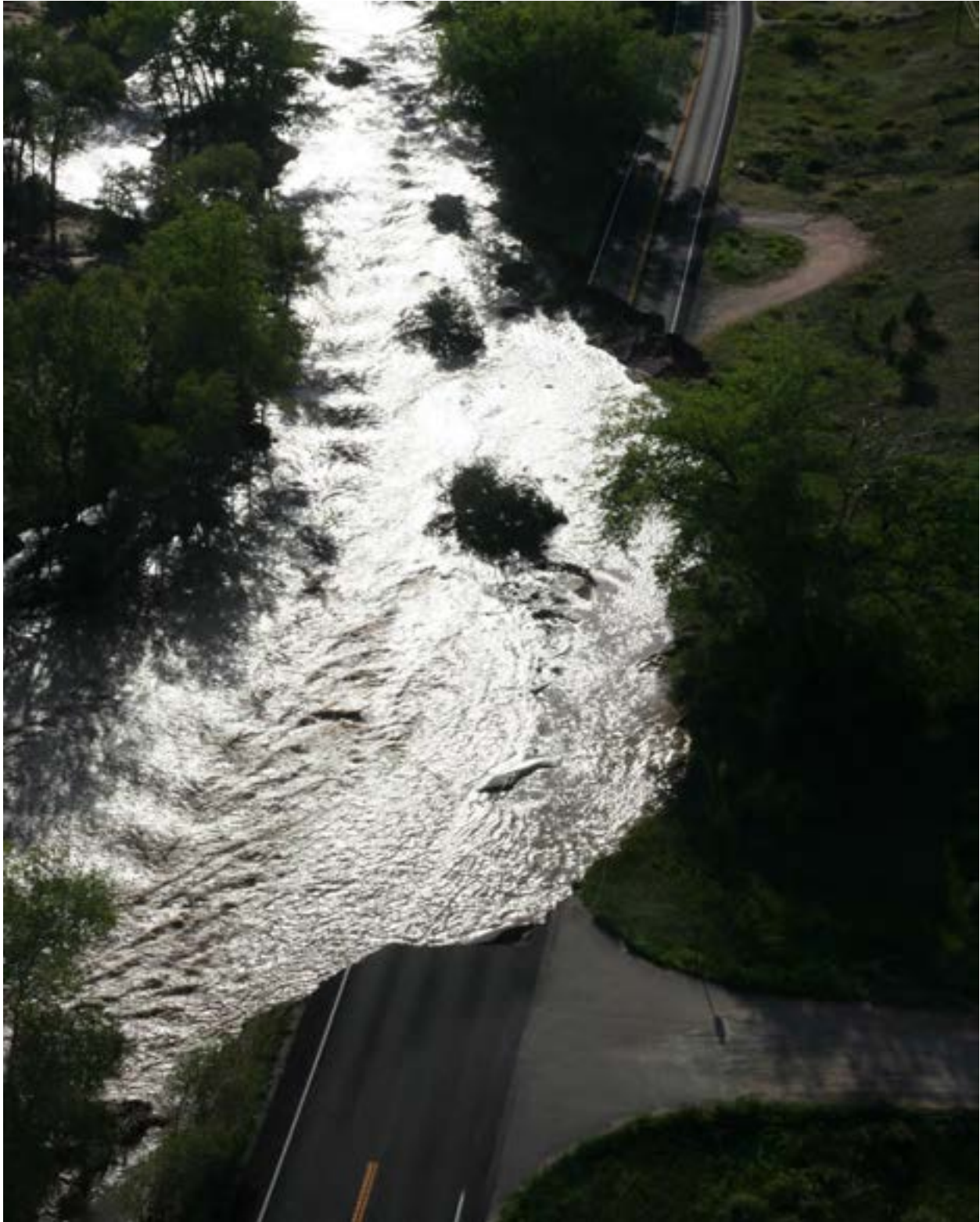
Figure 64 - MP 31.64, Complete loss of roadway.
