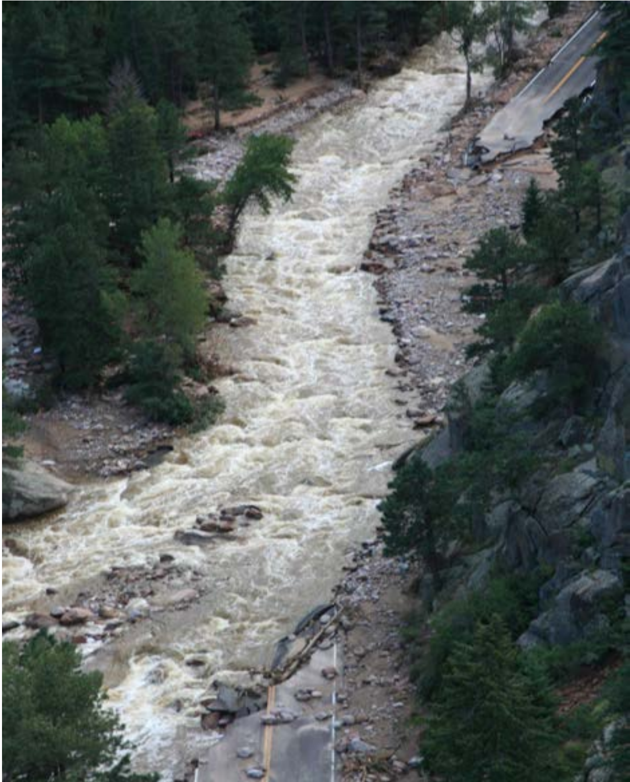
Figure 41 - MP 28.5, Complete wash out of the roadway due to lateral scour and overtopping of the roadway.
