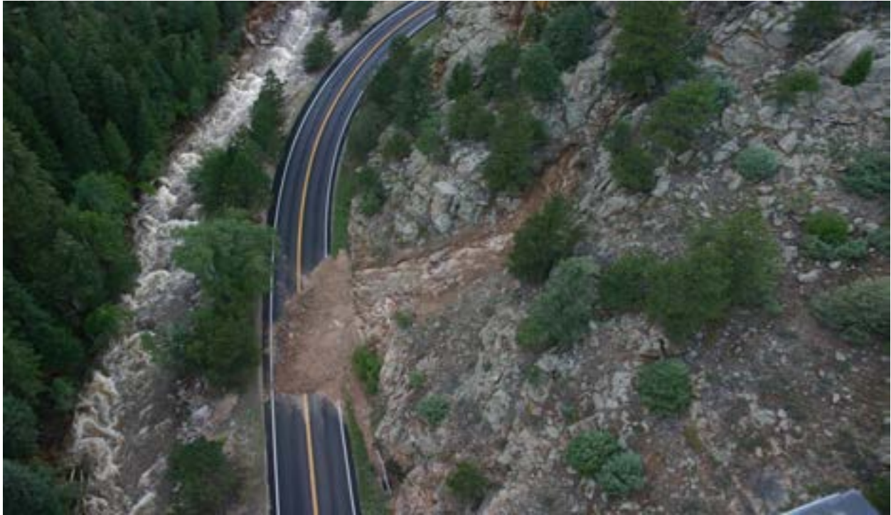
Figure 26 - MP 24.0, Rock slide covering both roadway lanes.
