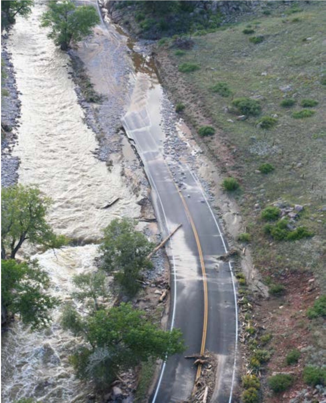
Figure 43 - MP 30.1, Wash out of the roadway embankment and pavement due to lateral scour and overtopping of the roadway. Sediment and debris deposition throughout.
