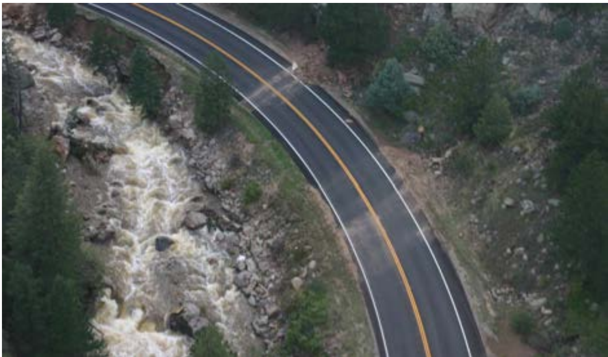
Figure 18 - MP 22.5, Riverside embankment loss and material slide onto the roadway.
