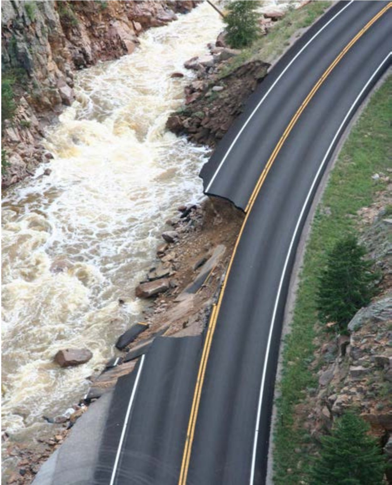
Figure 31 - MP 25.75, Embankment and partial roadway washout.
