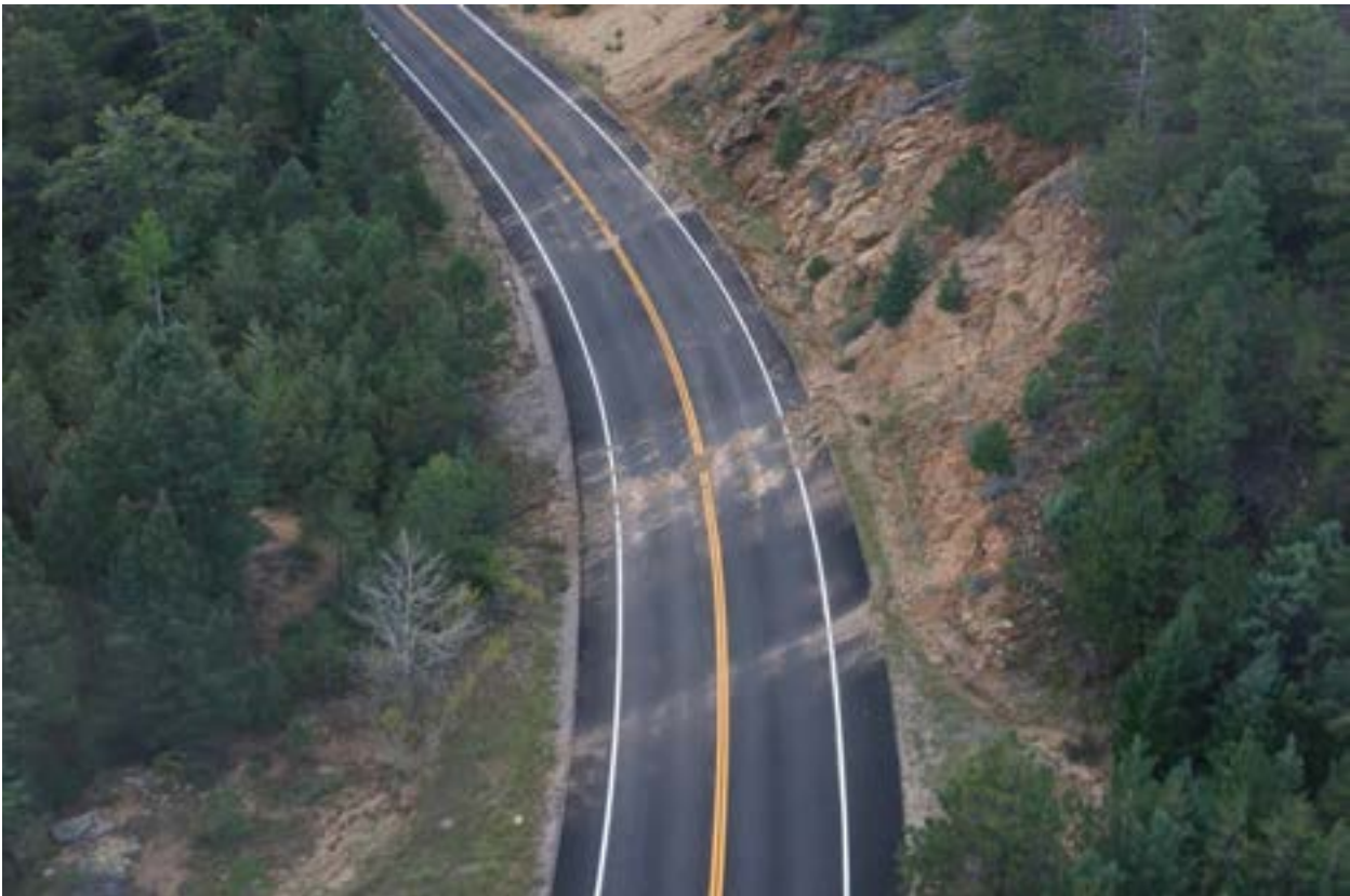
Figure 11 - MP 20.66, Westbound ditch damage and material slide.
