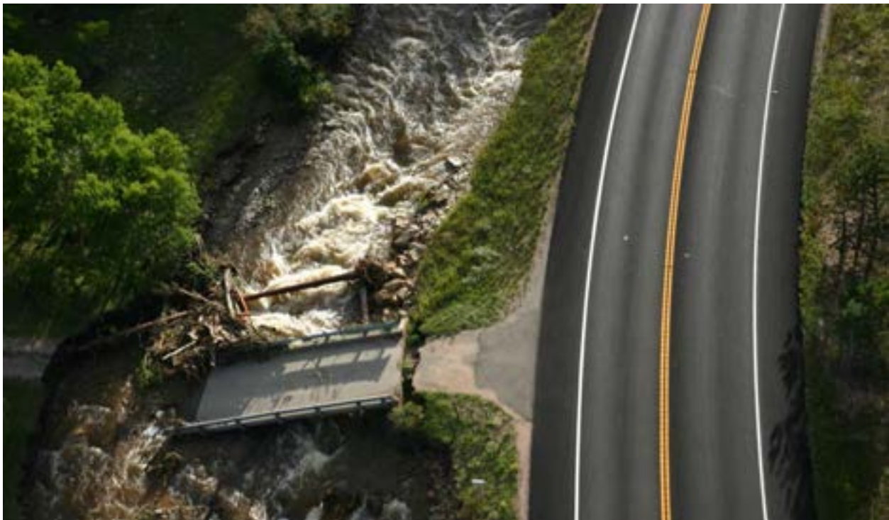
Figure 14 - MP 21.68, Local access bridge washed out and embankment damaged upstream and downstream of structure.
