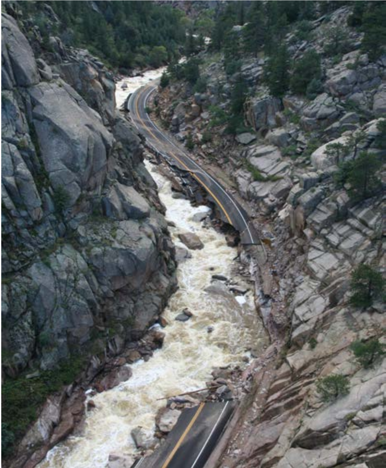
Figure 39 - MP 27.68, Wash out of riverside embankment and roadway due to lateral scour and overtopping of the roadway.
