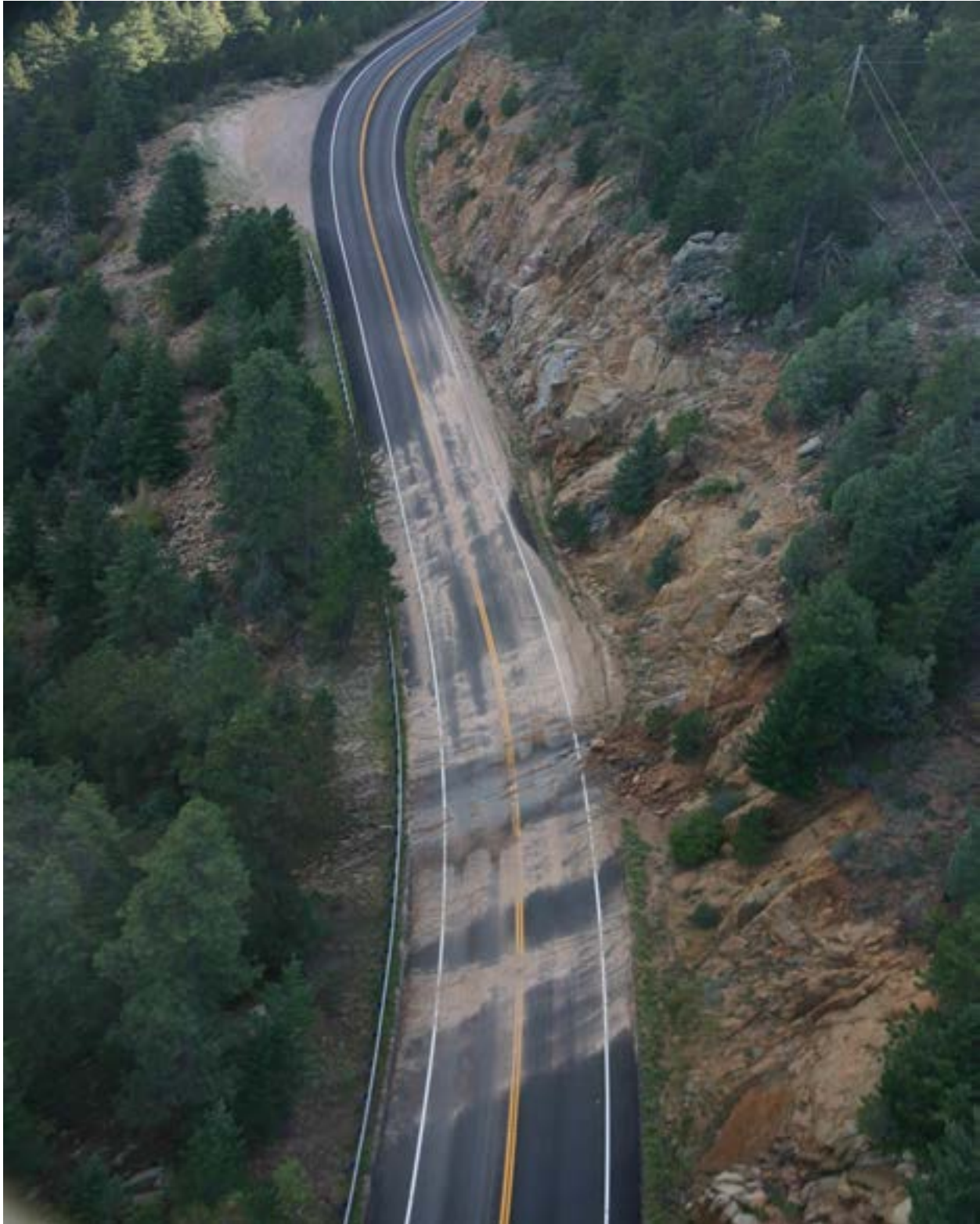
Figure 12 - MP 20.86, Material slide onto road.
