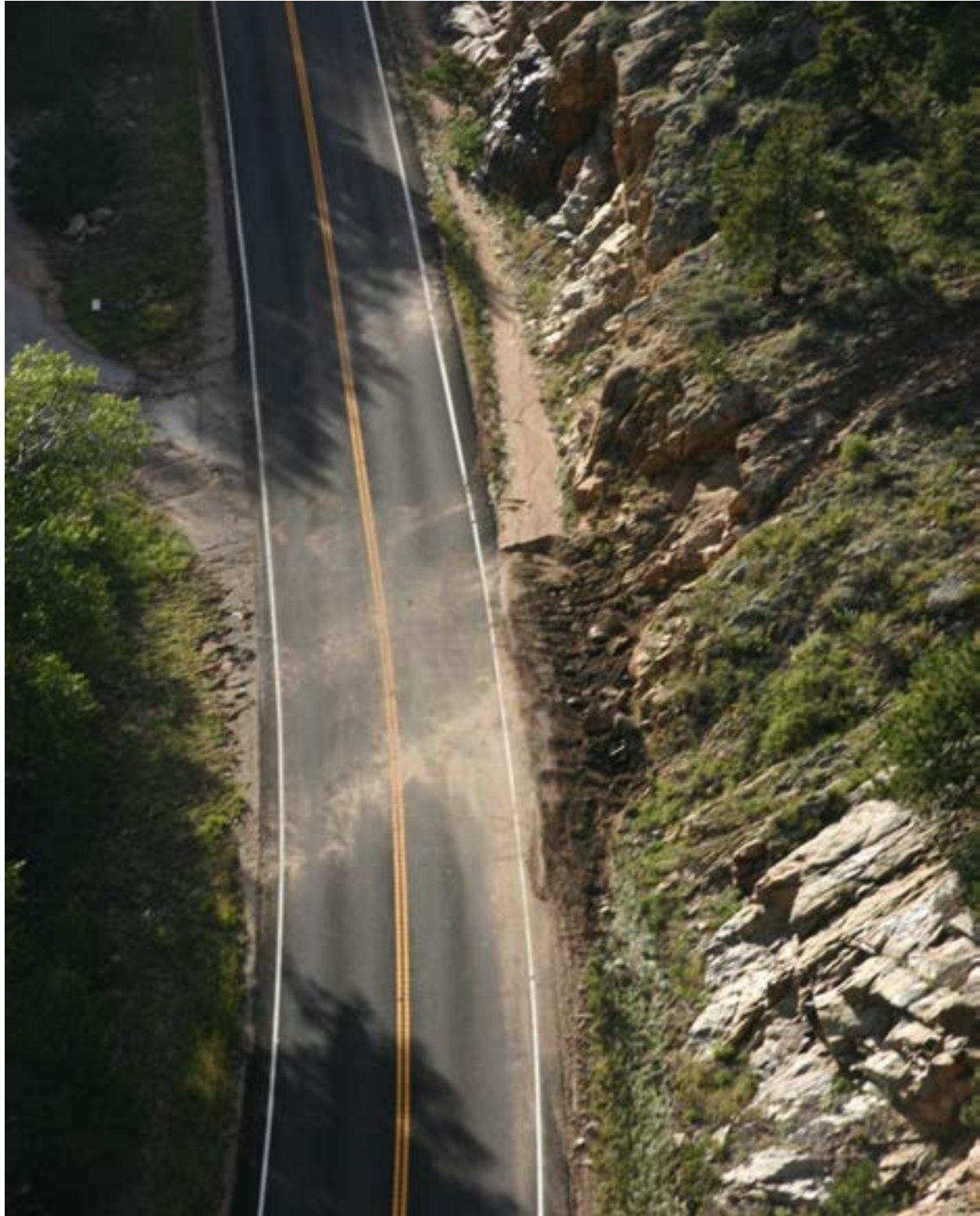
Figure 19 - MP 22.83, Material slide onto roadway.
