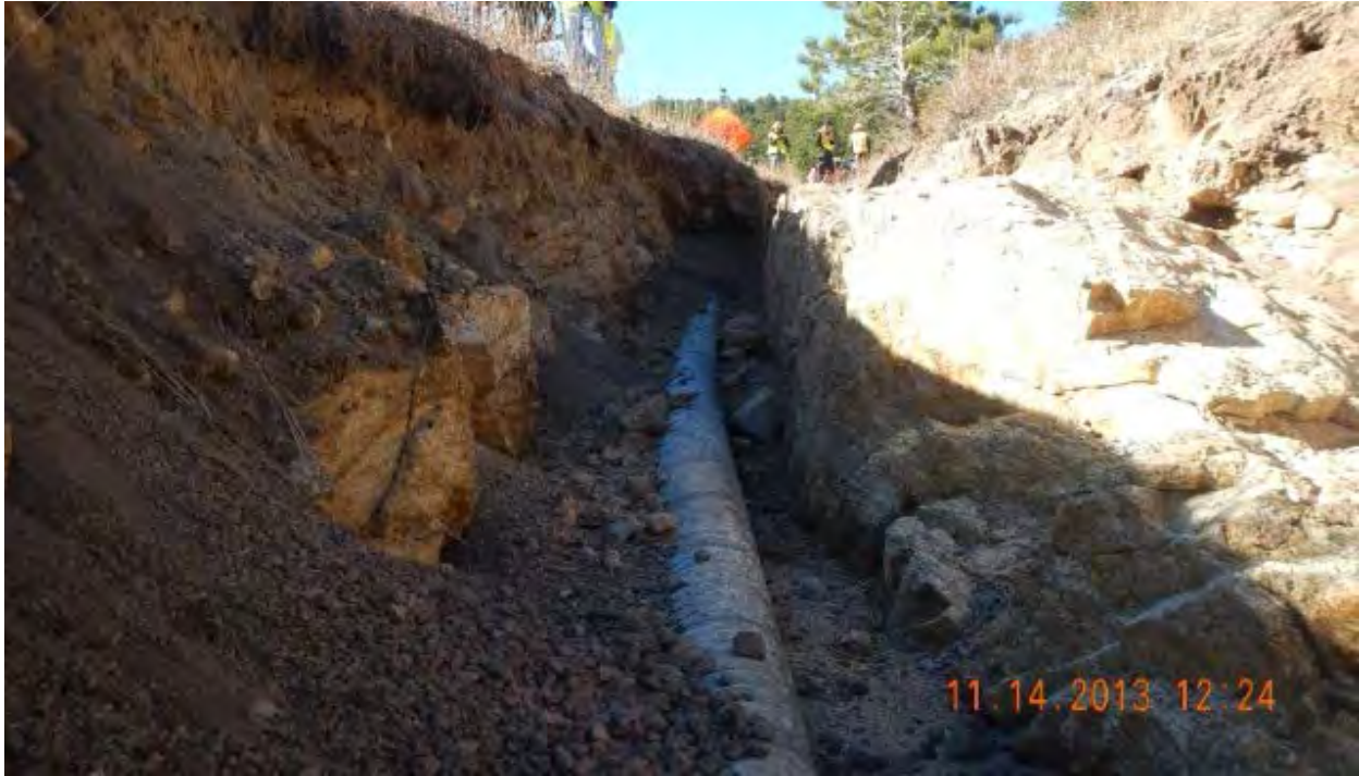
Figure 10 - MP 19.34, Westbound ditch damage.
