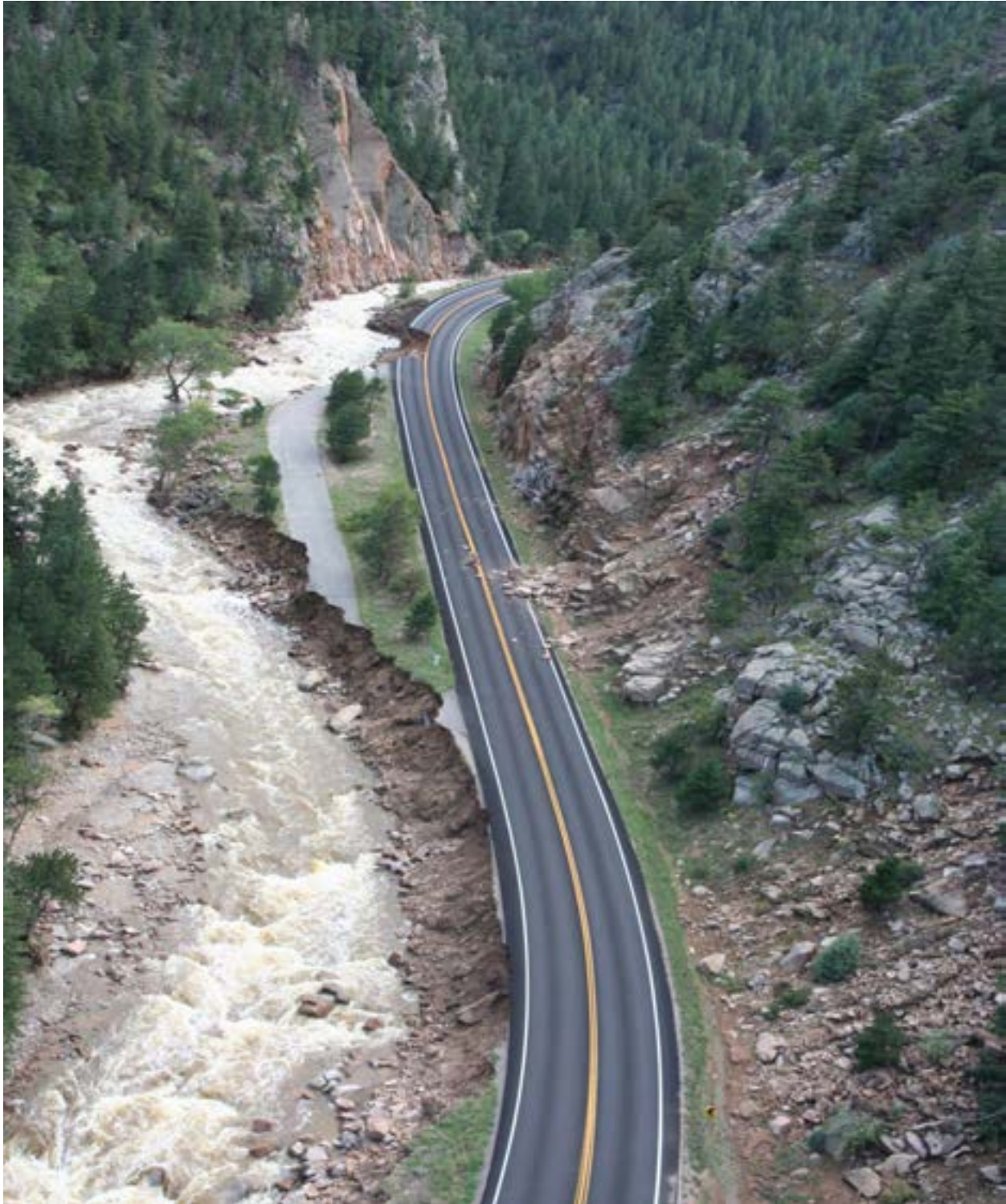
Figure 32 - MP 25.8, Embankment/pavement washout and rockslide.
