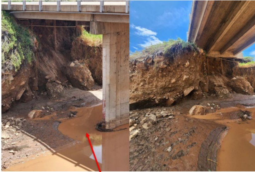
Figure 1 Original scour from washout event. Scour prism oval outline around Pier 1 is a textbook signature of pier scour footprint. Prior to the abutment failure, pier scour is suspected to have reached near the bottom of the pier footing prior to filling in with material from tailend of runoff surge.
