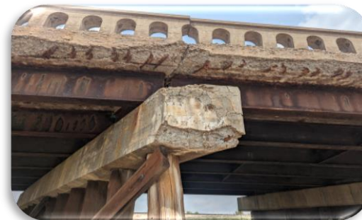
Deteriorated B-27-D Overhang and Pier Cap
