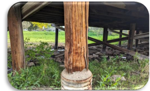
Splintering and Concrete Enclosed B-27-A Pile
