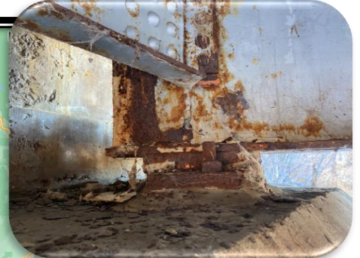
Repaired and Corroded K-09-B Bearings
