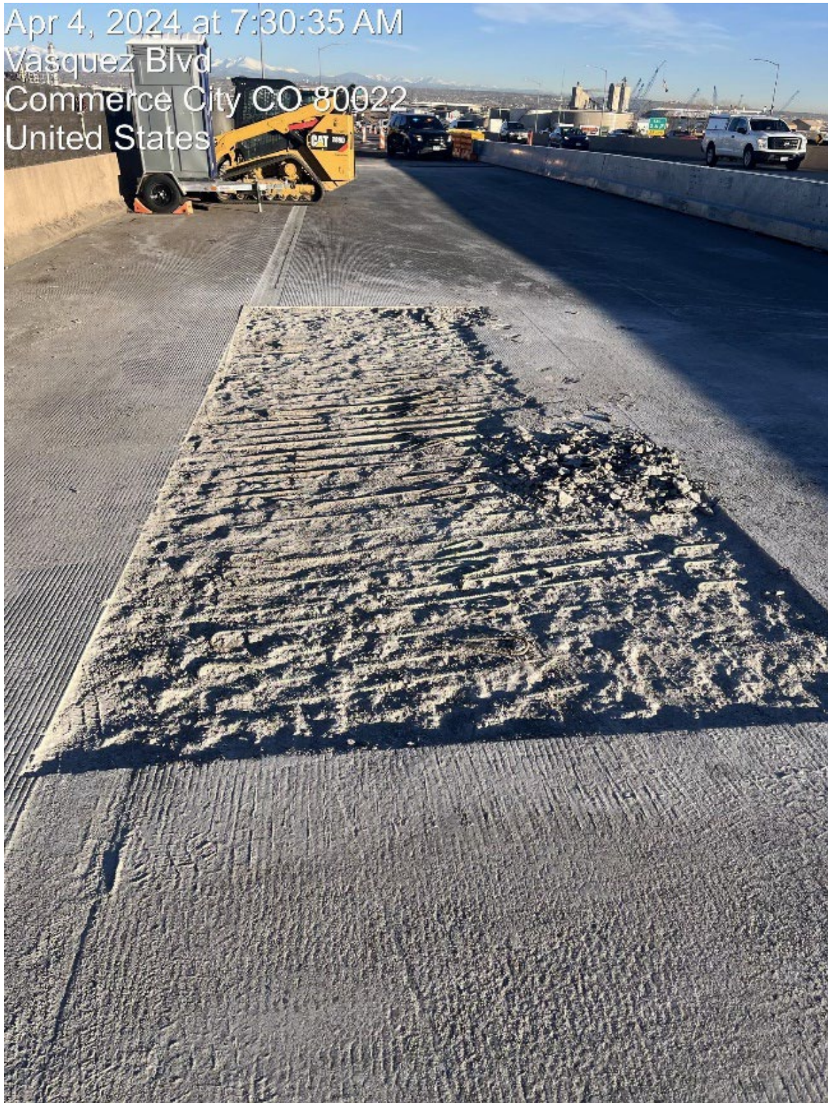
Figure 2- EB-270 over Vasquez showing exposed #4 transverse bars with approximately 1/2" of concrete cover. This is a good example of the surface condition that will exist prior to polyester overlay.
