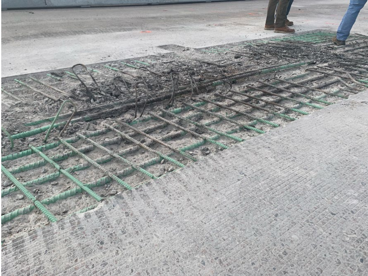
Figure 1- WB-270 over Vasquez showing removal below #8 longitudinal bars and resulting issues with concrete cover during pour back.
